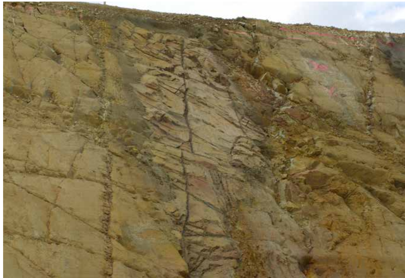
Fig. 6.33: Shotcrete finish to match adjacent rock (shotcrete section at centre of photo)
