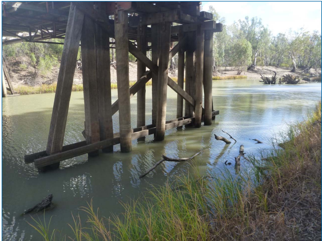
Photo 6: Woody debris under the bridge
