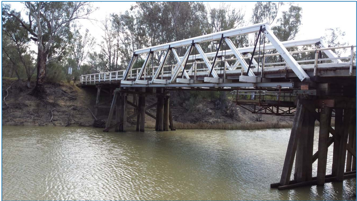
Photo 10: View of Gee Gee Bridge with the southern embankment in the background
