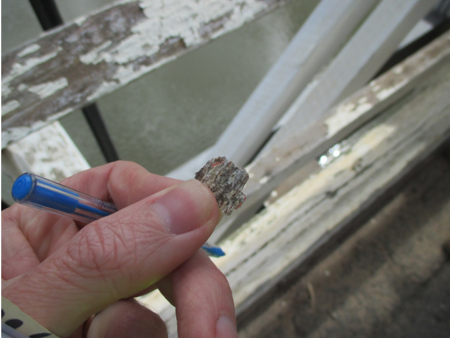
Plate 3 – Visual of Lead paint – posts, rails and kerbs
