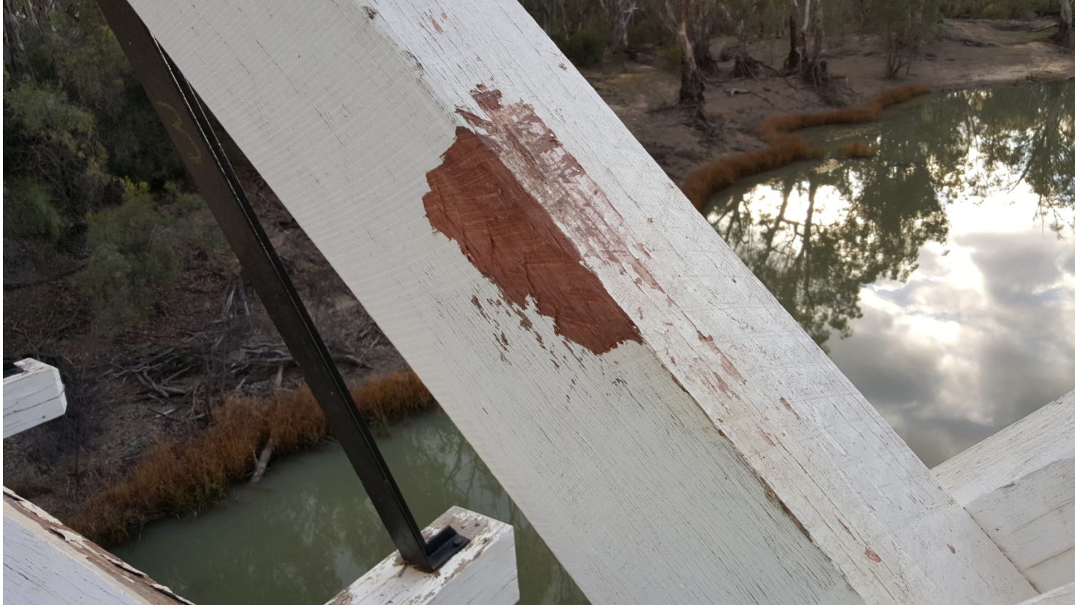
Plate 19 – Cross Members of Truss showing visual signs of lead paint
