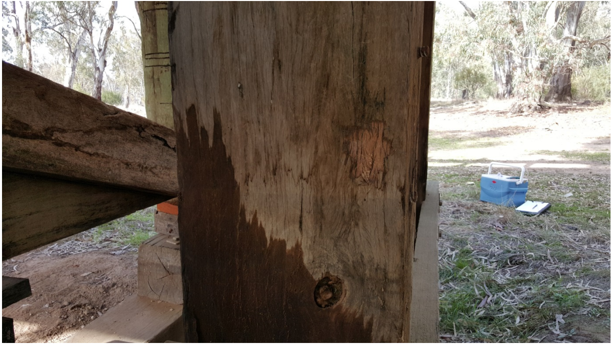
Plate 7 – Visual signs of contamination in Piles
