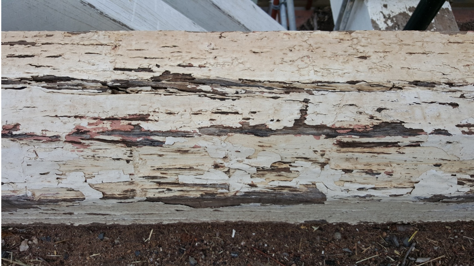
Plate 18 – Visual signs of Lead paint, western kerb
