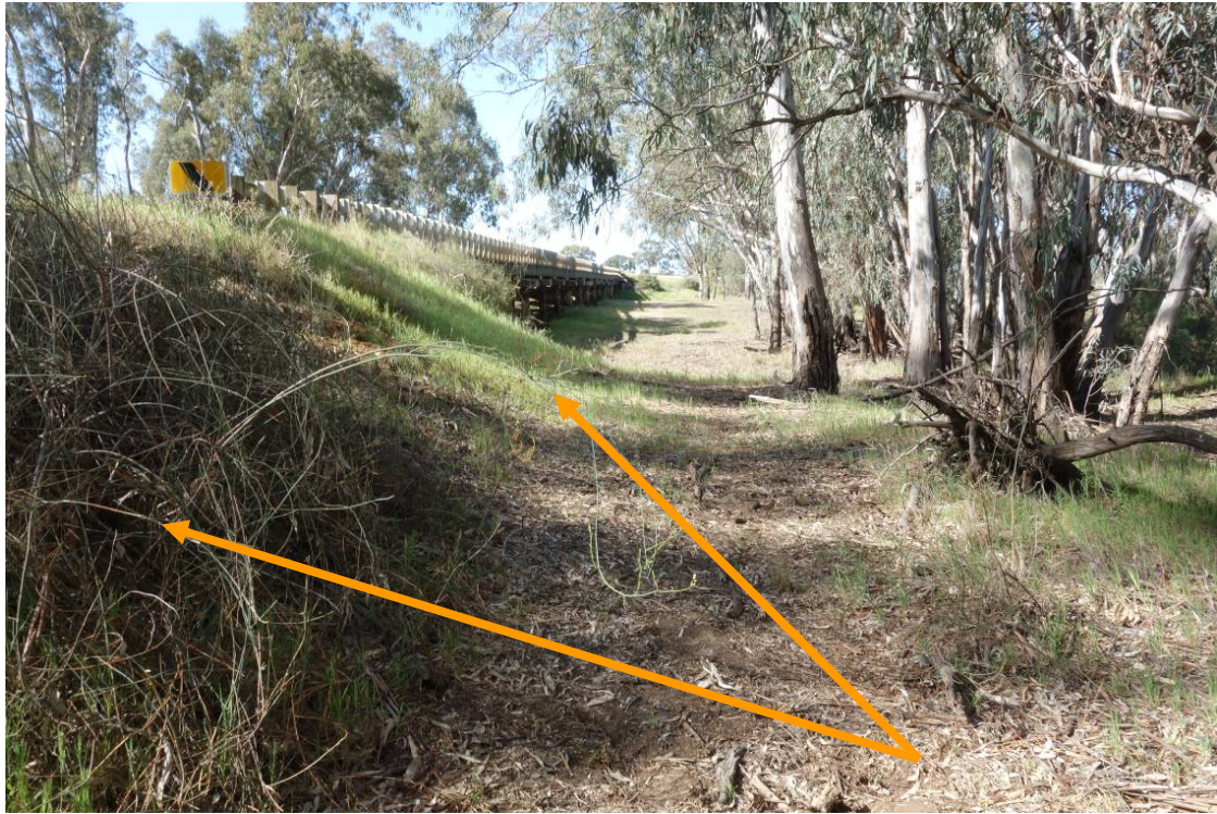
View Upstream of the road embankment between the two bridges - Remove road embankment to match existing natural level
