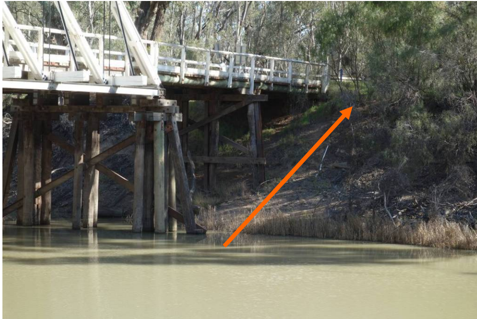
Main Channel Bridge - Swan Hill Approach Abutment – It appears that the abutment is located at the top of the river bank and too close to the river
