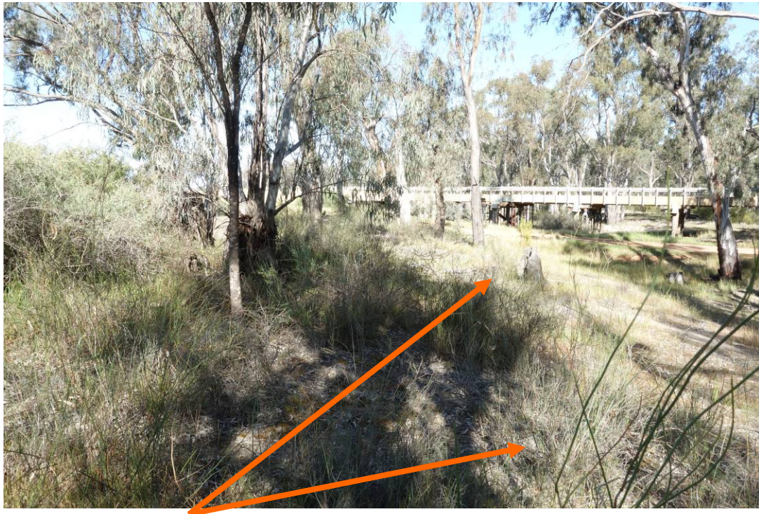
Flood Relief Approach Bridge – Downstream embankment in line with the bridge abutment on Wakool Approach
