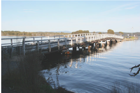
Wallaga Lake Bridge with up to 14 piles in some piers, representing 116 years of maintenance
