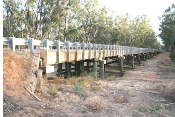
Gee Gee North Approach Bridge with concrete deck over timber, on heavily upgraded timber piers.
