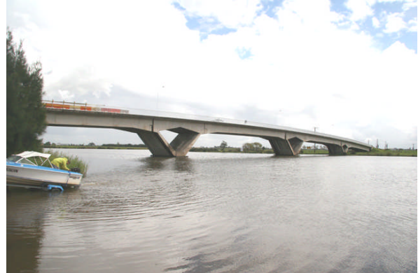
Fitzgerald Bridge with its unusual splayed piers and prestressed concrete beam deck
