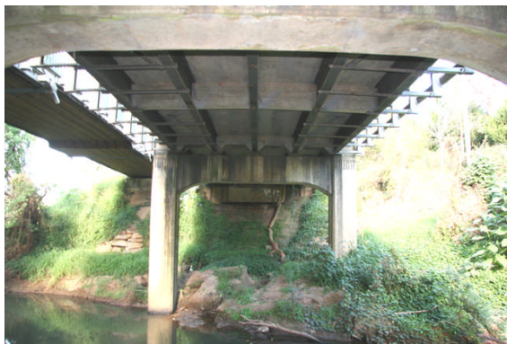
Red Bank Creek Bridge with steel beams visible. Cable stayed footbridge is to left
