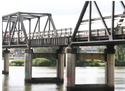
Through trusses and plate web girder of former lift span, Martin Bridge, Taree
