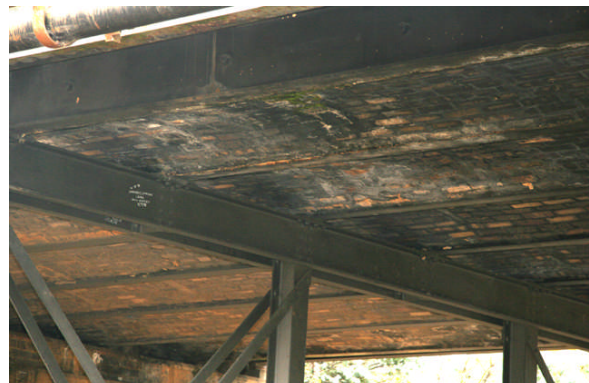
Railway Bridge at Armidale with brick arched deck support on steel beams (near bricks are soot stained from steam engines)
