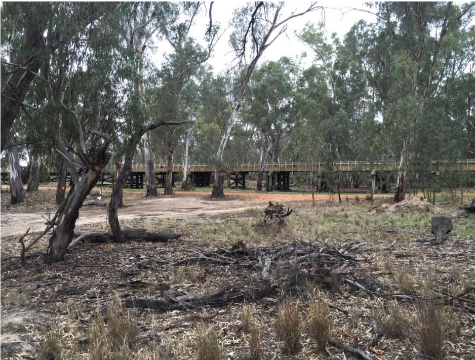
Figure 5.1 : Existing Gee Gee Bridge. The new bridge is proposed to be adjacent to this bridge (within 50 m), on the same side (north) as this photograph was taken (view south, photograph taken by Jeff Hill, 28 May 2015)
