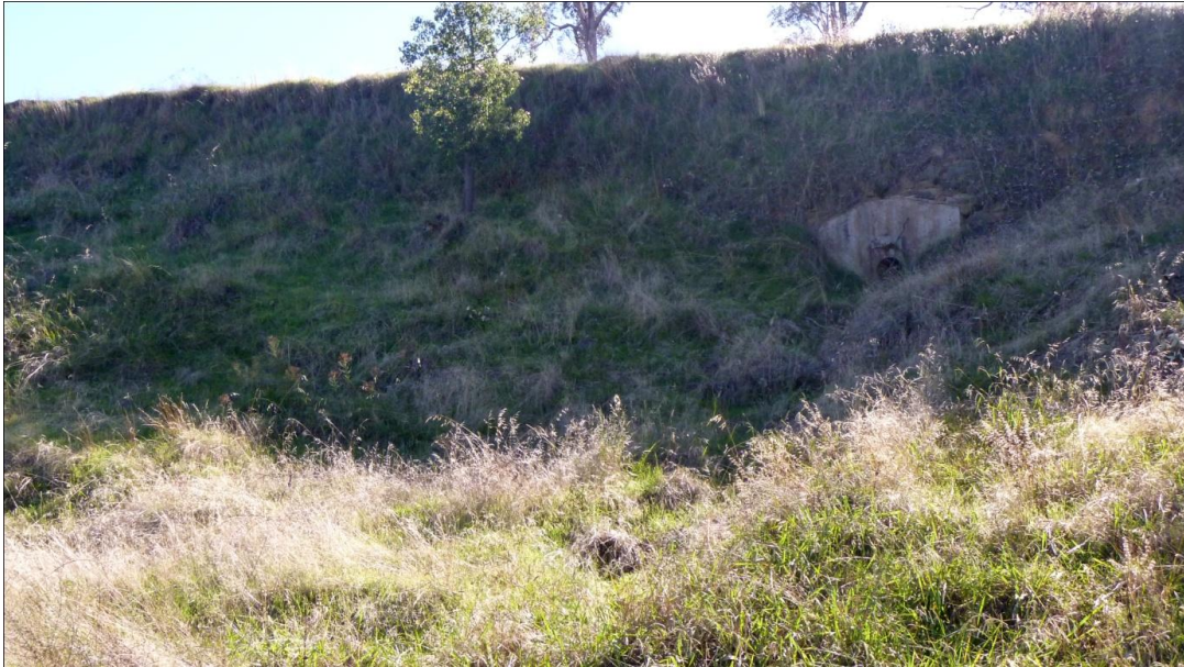
Figure 4.5: Detailed view of Item 2 small stone culvert formation (at right) taken from current road level and showing built-up road surface abandoned alignment.
