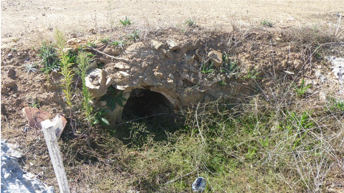
Figure 4.54: Detailed view of the remains of a stone rubble culvert and earthenware drainage pipe.
