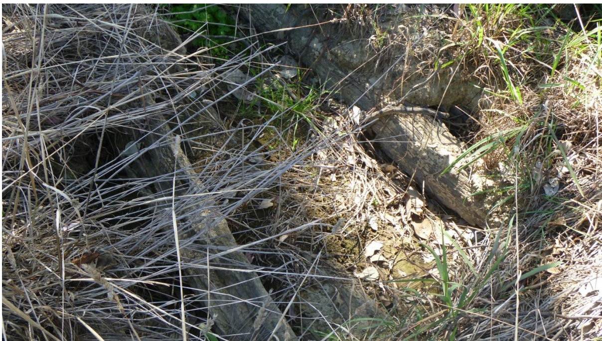
Figure 4.60: Detailed view of timbers the form the base of the crossing and the roof of the culvert.
