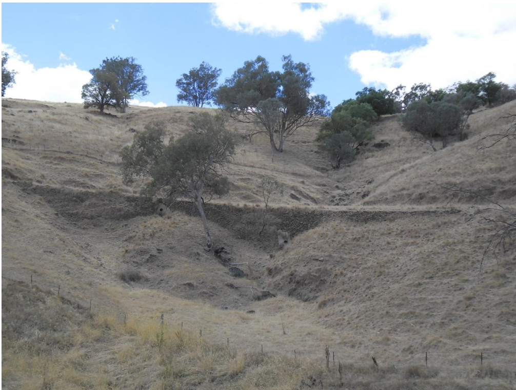
Figure 4.6: Detailed view of Item 3 large stone supported road formation showing concrete pipes and surface level of abandoned section of road spanning the drainage line.
