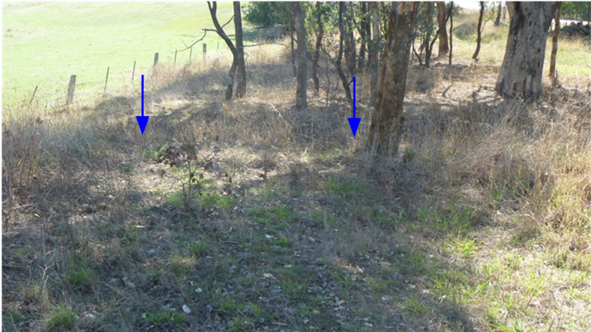
Figure 4.59: Context view of site of timber crossing in drainage line, looking north. The blue arrows indicate the total width of the crossing timbers.
