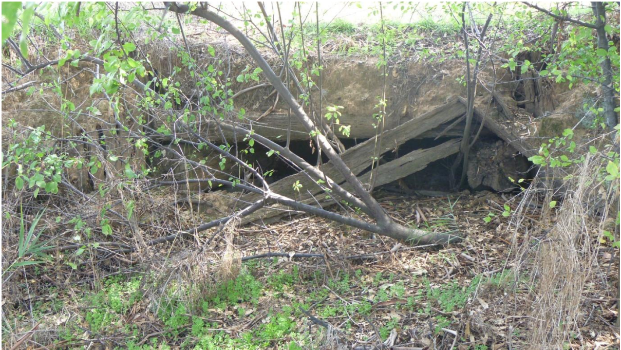
Figure 4.21: Timber crossing/culvert, looking south-west, showing the north-eastern alignment of the former road. Note the substantial bed logs, timber girders and timber wing walls. Note also the depth of coverage of stone and clay to form the road surface.
