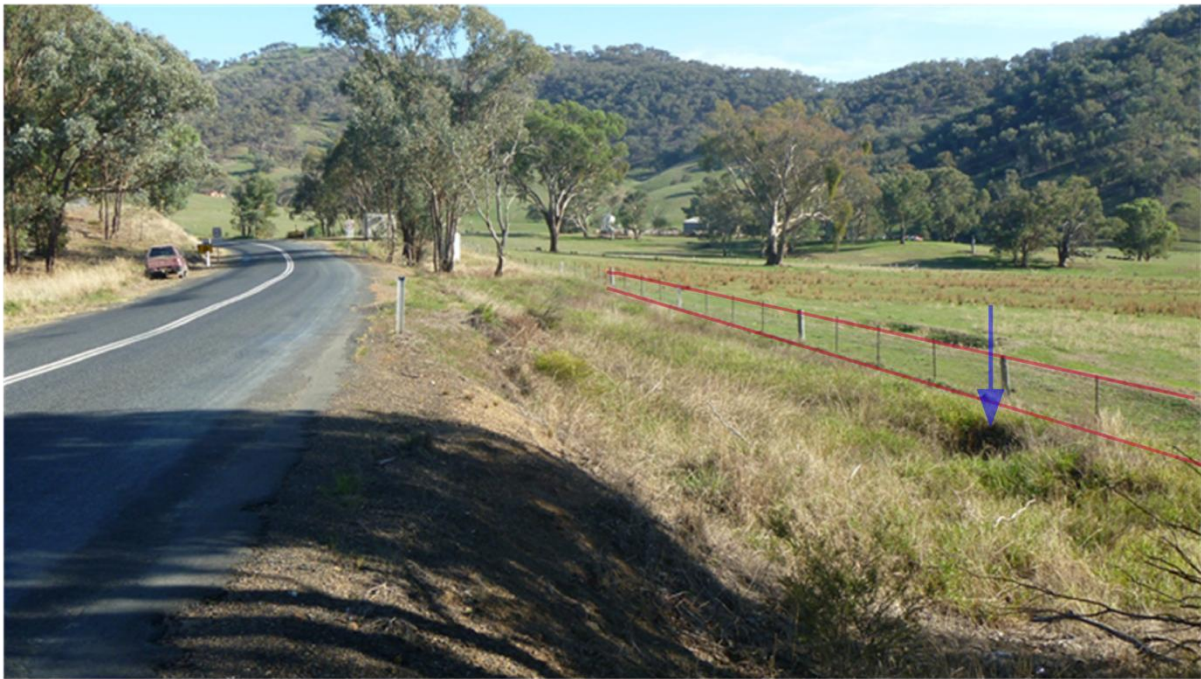
Figure 4.18: Context view of stone culvert looking north, with blue arrow indicating its position. The red overlay indicates the line of the old road surface.
