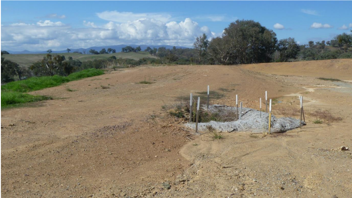
Figure 4.53: Context view of protected culvert formation with the old road formation just discernible to the left.
