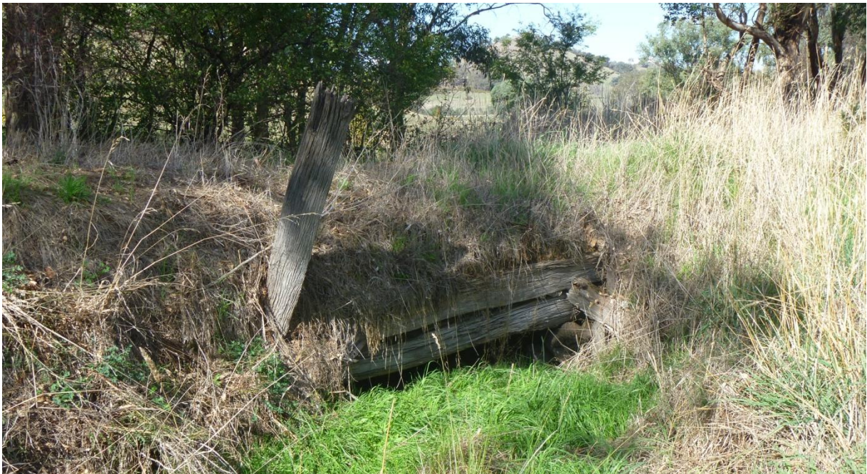
Figure 4.22: View of the south-western alignment almost obscured by grass cover. The timber culvert is still functioning as a drainage line. A single upright timber of the safety rail remains.
