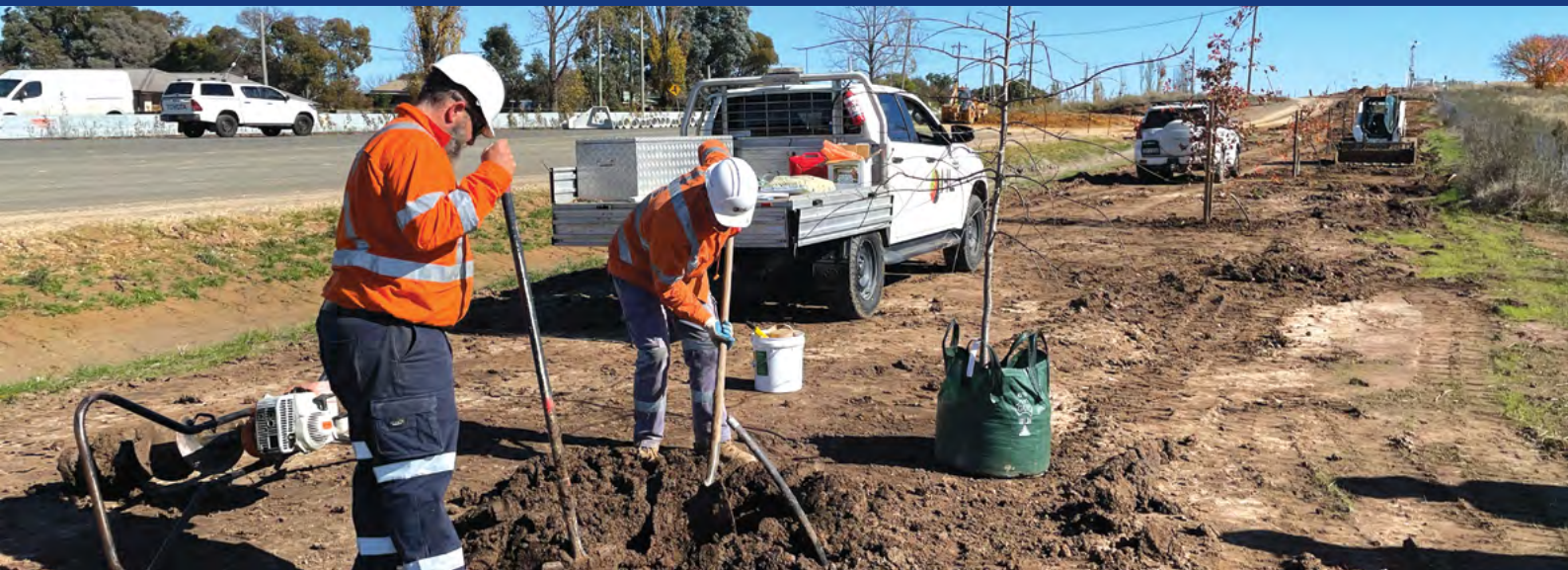
Landscaping taking place along the northern side of the Great Western Highway at Raglan.
