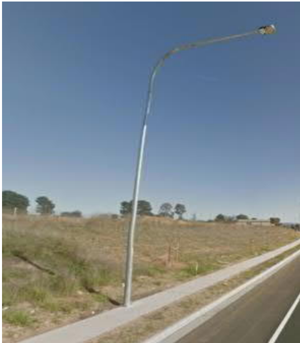
Figure 4-12 Typical overhead lighting at Kelso
