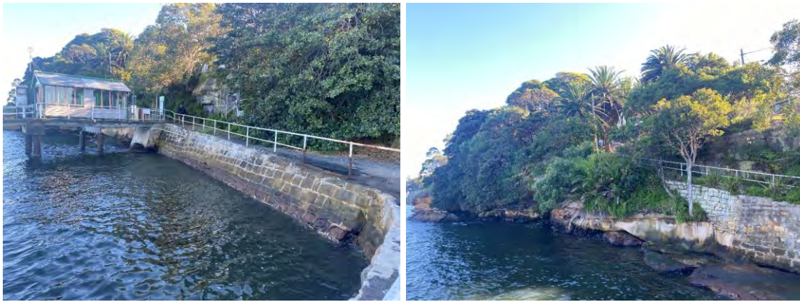
Figure 3-1: The sandstone seawall to the south-east (left) and north-west (right) of the existing wharf
