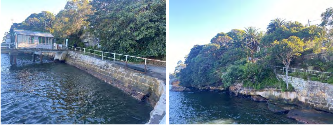
Figure 3-1: The sandstone seawall to the south-east (left) and north-west (right) of the existing wharf
