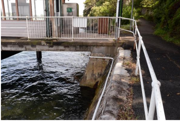
Figure 32: North-west view of the concrete wharf landing attached to the sandstone sea wall
