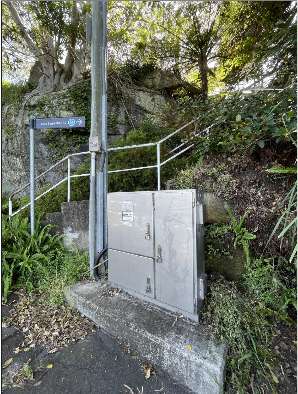
Photograph 5: Electrical services unit in front of the stairs.
