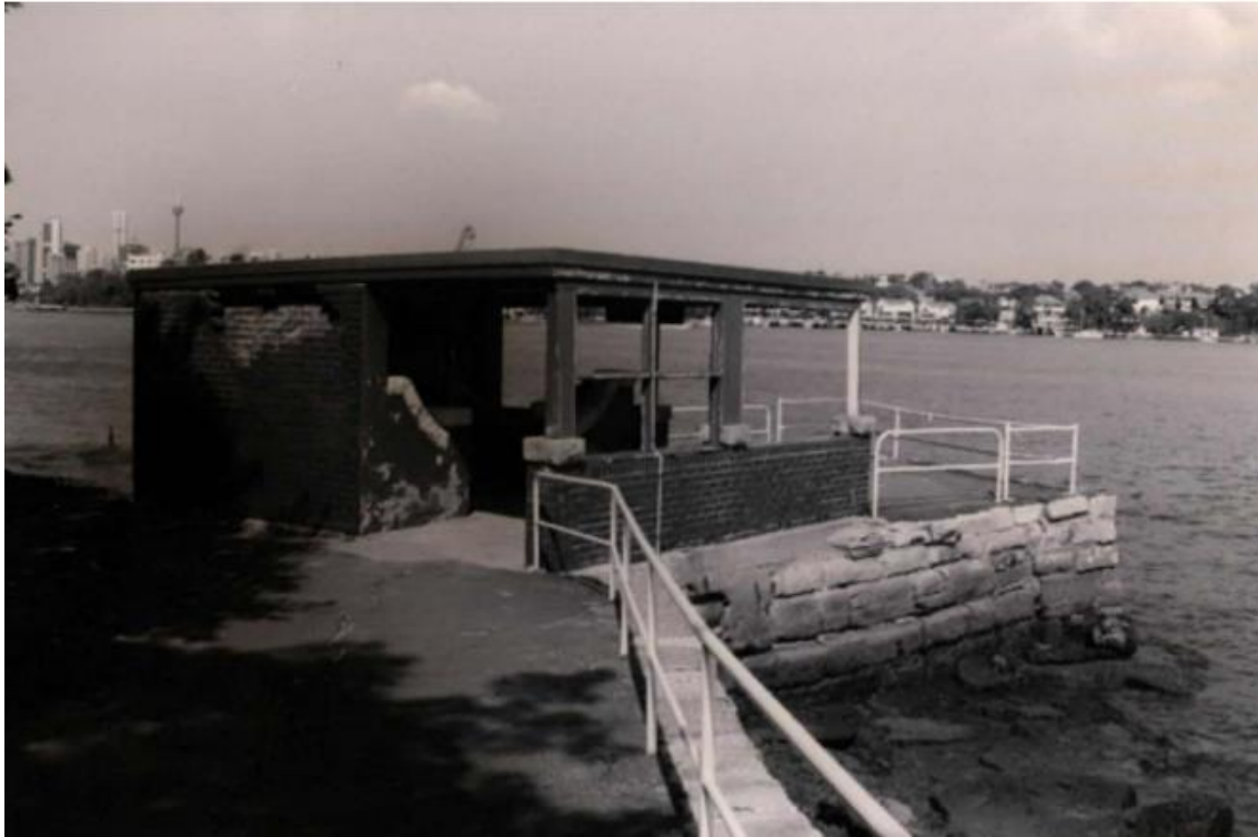
Figure 25: Close up of the Greenwich Point Wharf showing the deteriorated condition (window glass no longer present). Source: Sydney & Middle Harbours Heritage Study, GML, 1991.
