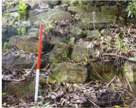
Figure 23: Sandstone retaining wall section within the south-western portion of the study area, adjacent to road corridor, facing east (Source: Biosis, 2020).
