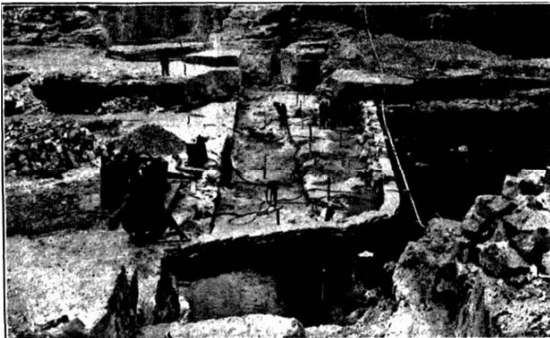
Figure 17: Kolara Weir's construction, 1931 (Source: 'Site of Weir on Woronora River', Construction and Real Estate Journal, 11 March 1931).
