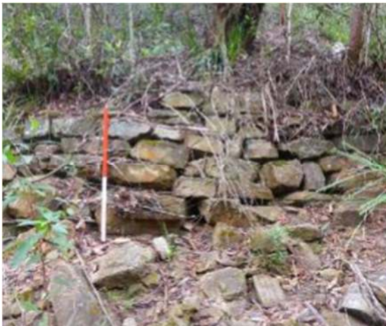
Figure 28: Small sandstone wall located adjacent to Heathcote Creek, most likely associated with the Weir (Biosis, 2020).
