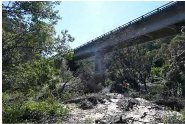
View 07 Close up view of the structure looking from the southern foreshore to the northeast. Note the structure being in the shade (dark grey) helping it to visually blend with the backdrop.
