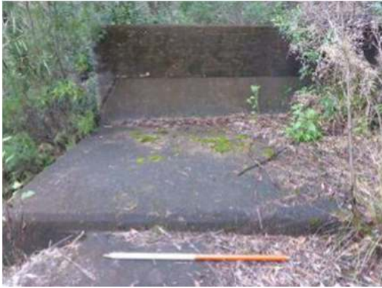
Figure 26: Large concrete material associated with the Weir in the north-western portion of the study area (Source: Biosis, 2020).
