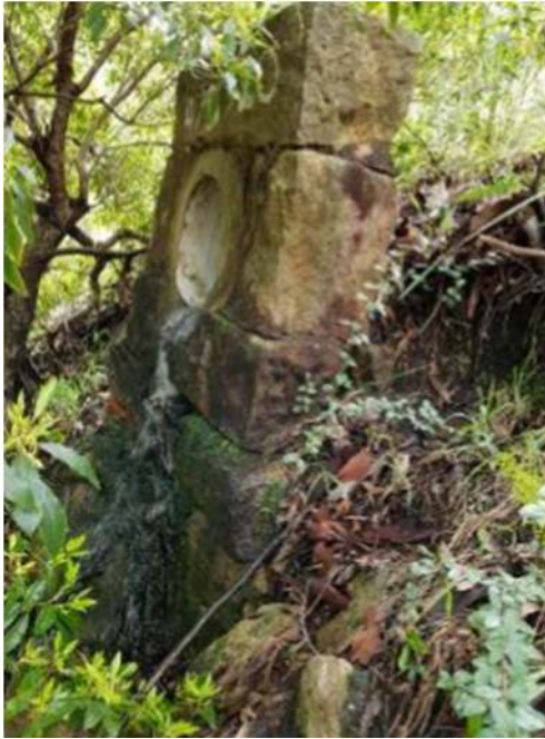
Figure 22: Example of sandstone culvert headwall with reinforced concrete pipe (culvert no. 475320) along south-western road alignment, facing north (Source: Biosis, 2020).
