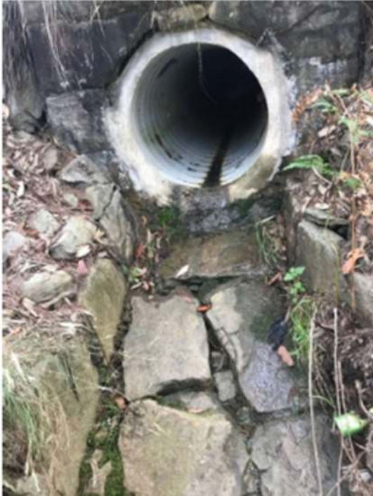
Figure 34: Outlet for Cross Drain Exist-01, provided by Fulton Hogan.
