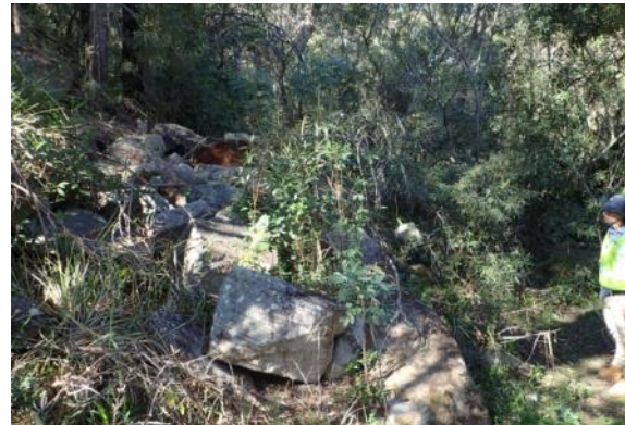
Plate 6. Facing south on the south western side of bridge. Note disturbed embankment between Heathcote Road and Heathcote Creek.
