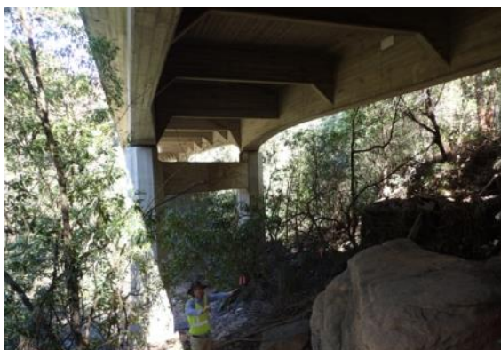
Plate 9. Facing south, beneath bridge. Note rocky slopes on northern side of river, these have been disturbed by previous road and bridge construction.
