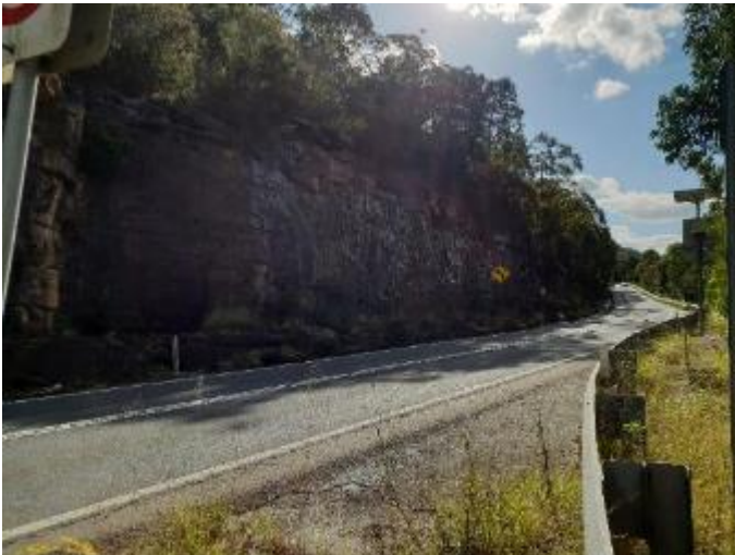
Photo 25 Example of the road surfaces and guardrails along Heathcote Road [4] visible throughout the study area, facing north
