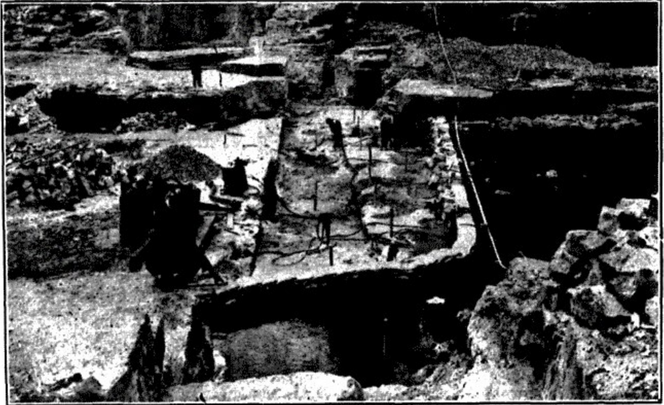
Photo 7 Kolara Weir being constructed in 1931 (Source: 'SITE OF WEIR ON WORONORA RIVER' Construction and Real Estate Journal (1930-1938) 11 March 1931, pp. 4)
