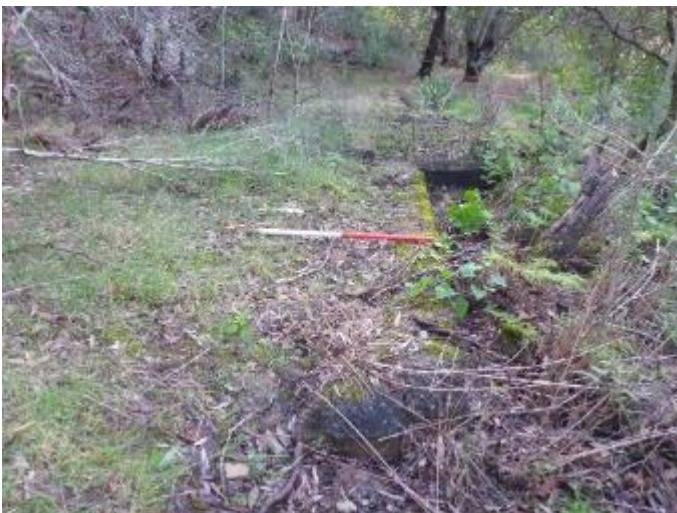
Photo 31 Concrete foundations located in the north-western portion of the study area, most likely associated with the Kolara Weir and the amenities block [8], facing north-west
