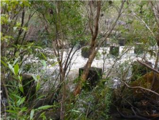
Photo 32 Concrete piers across the extent of Heathcote Creek, associated with the access track [6] and former bridge [7], facing west
