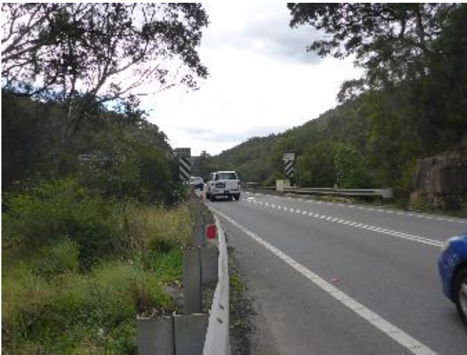
Photo 37 View of 1990 additions to Woronora River Bridge [5] comprising jersey kerb and rectangular steel rails on the southern approach, facing north
