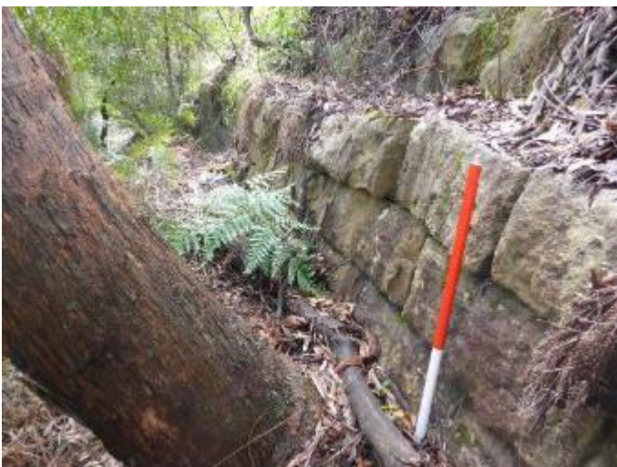
Photo 28 Well-constructed sandstone retaining wall section within the south-western portion of the study area, underneath haphazard retaining wall, facing north-east
