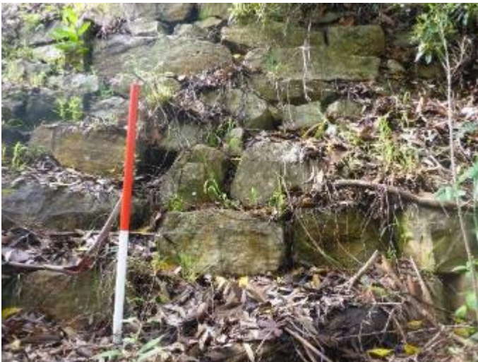
Photo 27 Sandstone retaining wall section within the south-western portion of the study area, adjacent to the road corridor, facing east
