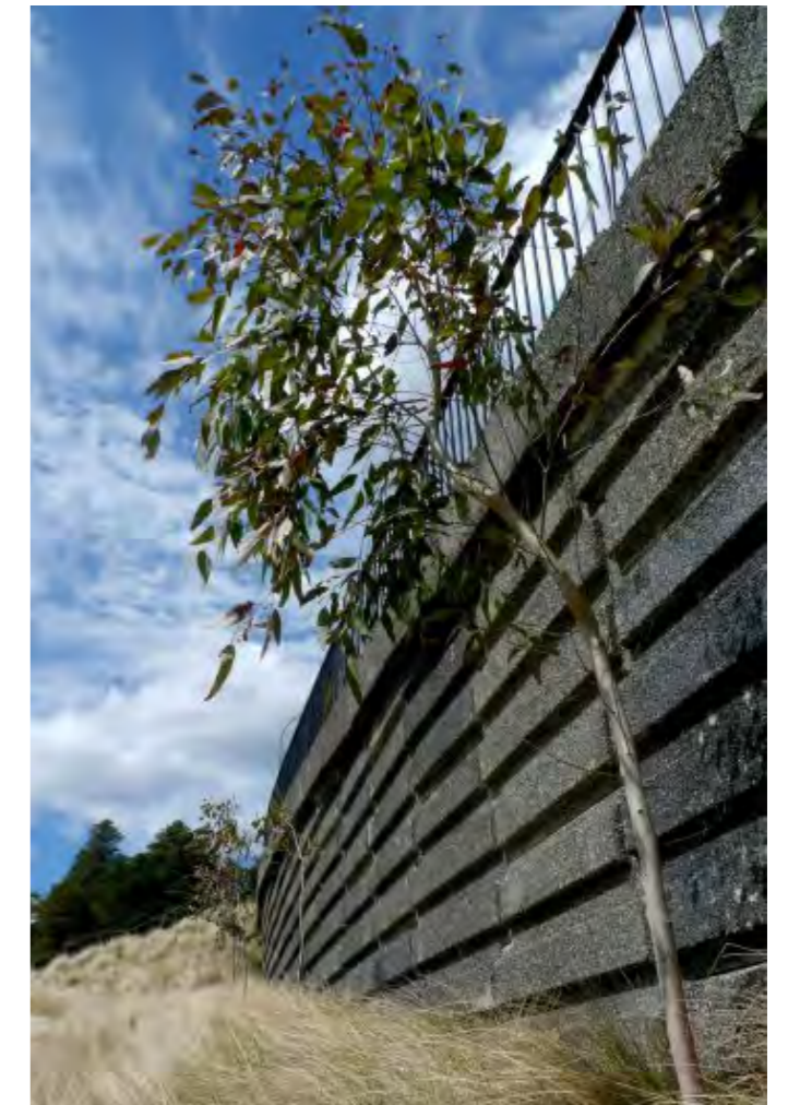
Figure 5.11 Example of a retaining wall in Leura, Blue Mountains, using oxide and an exposed aggregate finish to create a darker effect.
