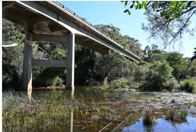
Figure 6.8 View looking north from the river foreshore with the structure clearly visible.
