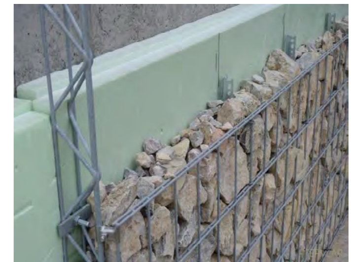
Figure 5.14 Example of a gabion cladding configuration. A similar approach is proposed for the abutment walls.
