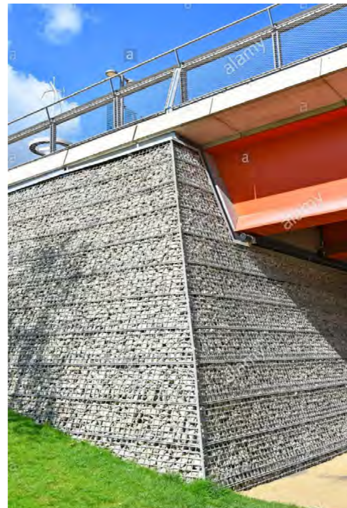
Figure 5.9 Example of a bridge abutment using gabion baskets, giving the structure a more naturalistic character.
