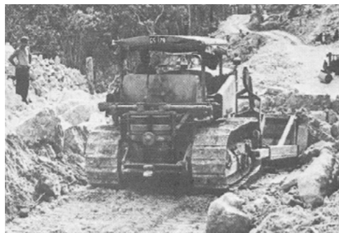
Figure 2.5 Heathcote Road being constructed in 1941. Source: Bridge over Woronora River near Heathcote - SOHI Report | October 2020
