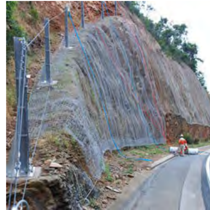
Figure 5.18 Example of a rock mesh/rockfall barrier.
