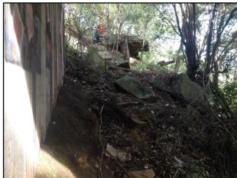
Material waste beneath bridge abutment (southside facing south)
