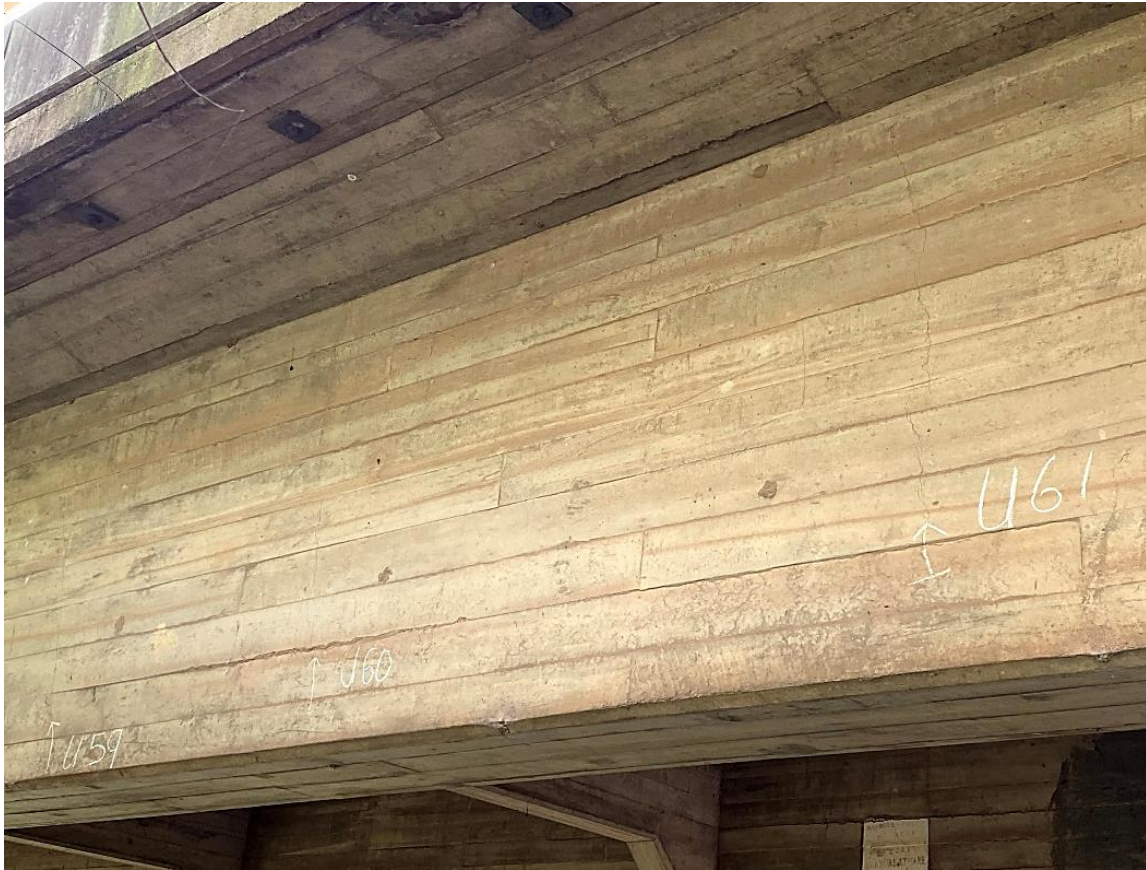
Figure 2-5 Photo of fine cracks (marked with U59, U60 and U61) under the bridge
