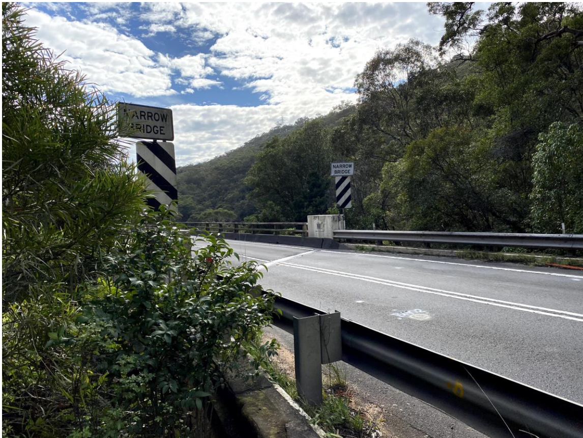
Figure 2-3 Photo showing narrow lanes and shoulders on Heathcote Road bridge
