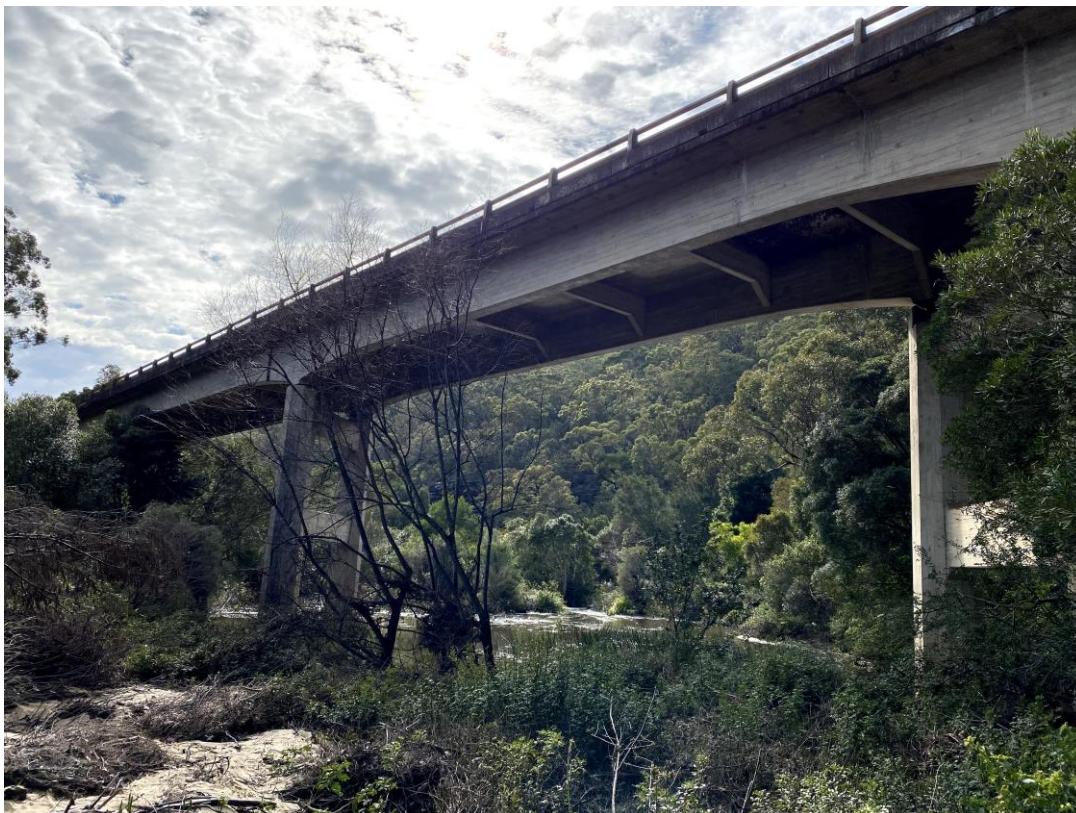
Figure 3-6 Photo showing existing Heathcote Road bridge structure from underneath and steep river valley surrounding Woronora River
