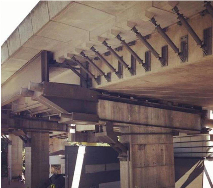
Figure 2-10 Example of bridge widening where a combination of headstock extension and steel bracket widening methods have been used from Market Street viaduct widening in Darling Harbour
