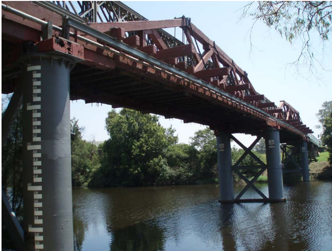
View of the timber trusses, members under the bridge and the cast iron piers
