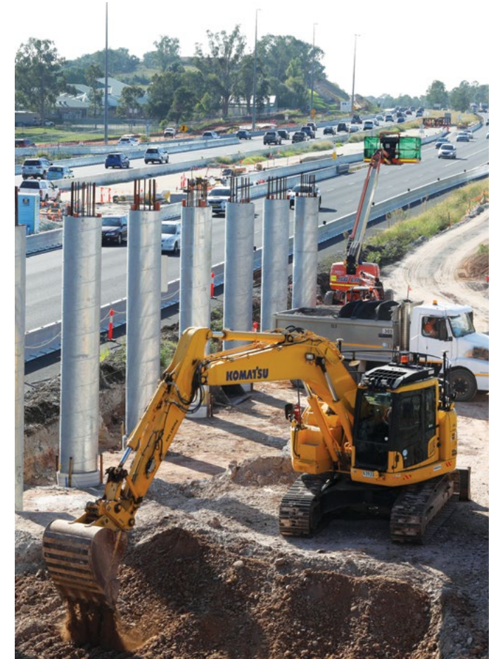
Construction of the columns for the southern abutment of the new bridge
