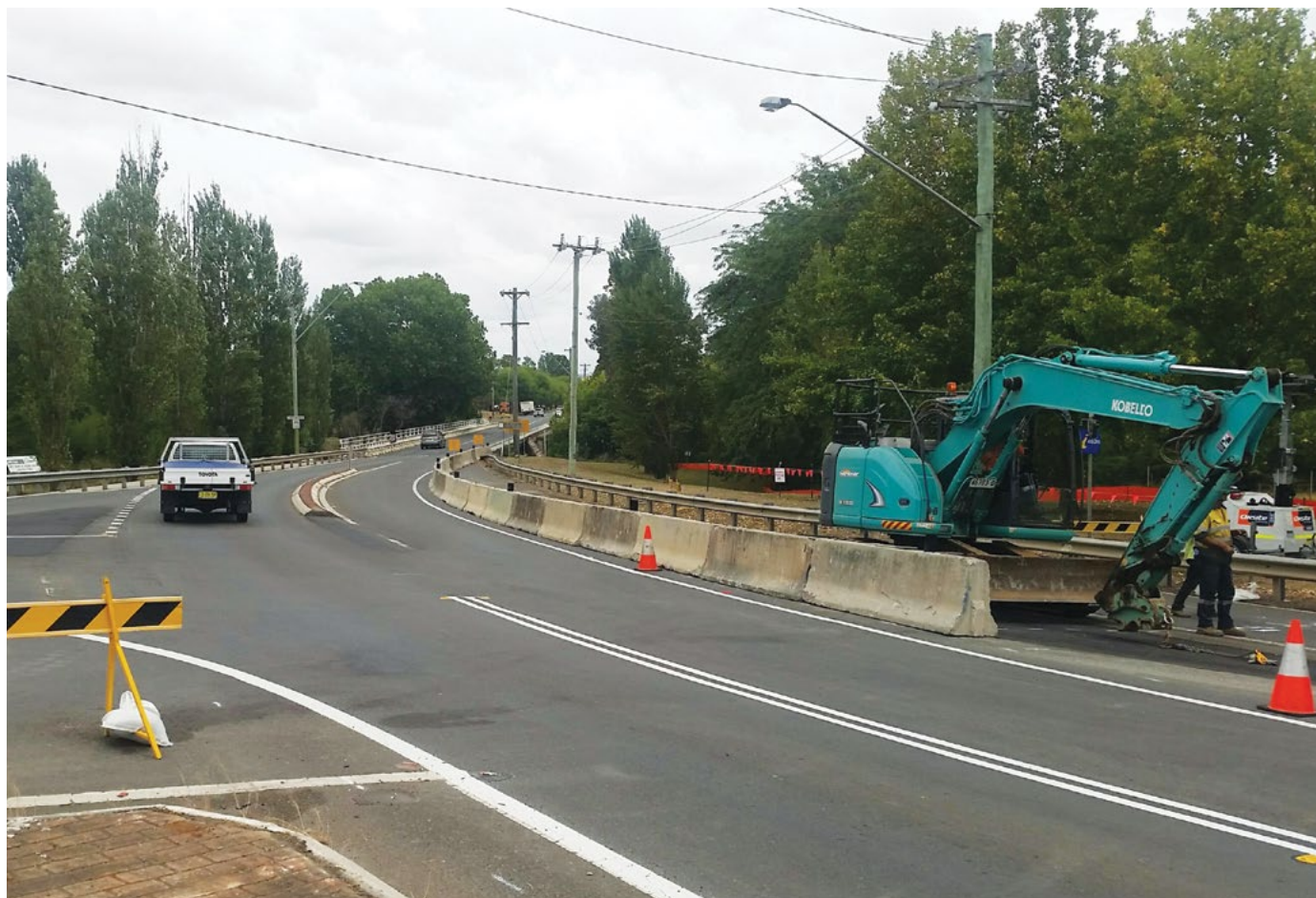
Camden Valley Way/Macarthur Rd Intersection upgrade - Preparation work for utility adjustments on Camden Valley Way eastbound.
