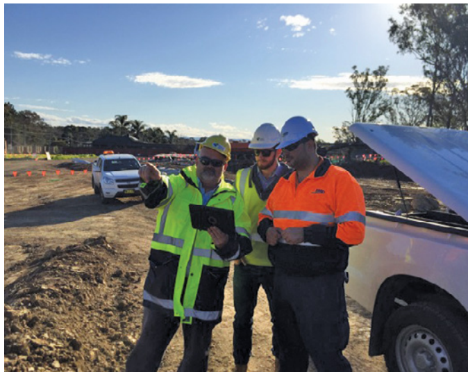
Roads and Maritime staff doing a safety inspection of a bridge at the Bringelly Road site
