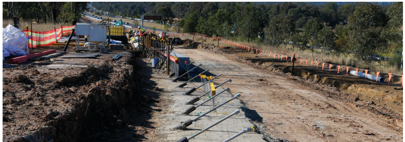
Construction of the new soil nail wall, retaining wall and ramp to the M4 at the Werrington Arterial Road site
