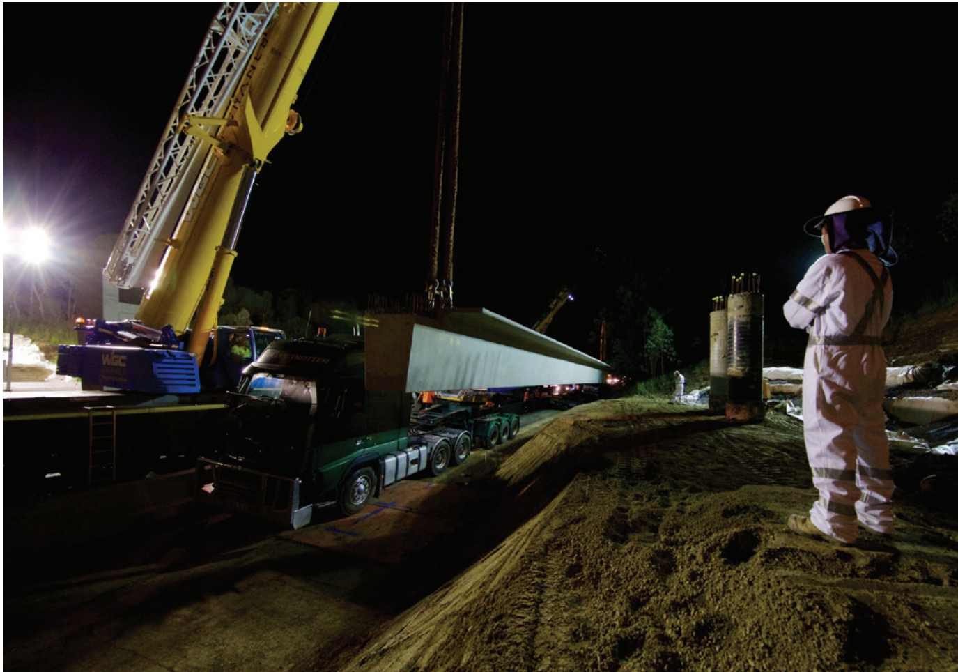
Delivery of girder for new shared pedestrian and cycle bridge across M4 Motorway
