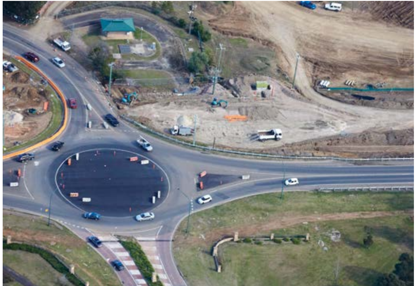
Roundabout at The Northern Road and Fairwater Drive/Porrende Street, Harrington Park looking west
