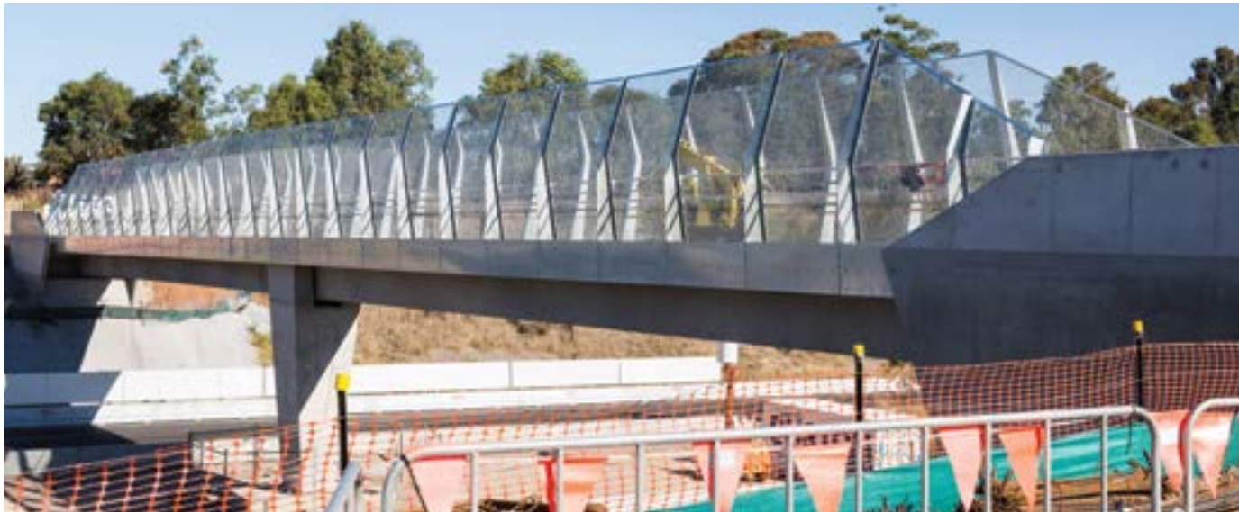
Werrington Arterial Road new shared pedestrian pathway over the M4 Motorway west of the Kent Road Bridge, Claremont Meadows
