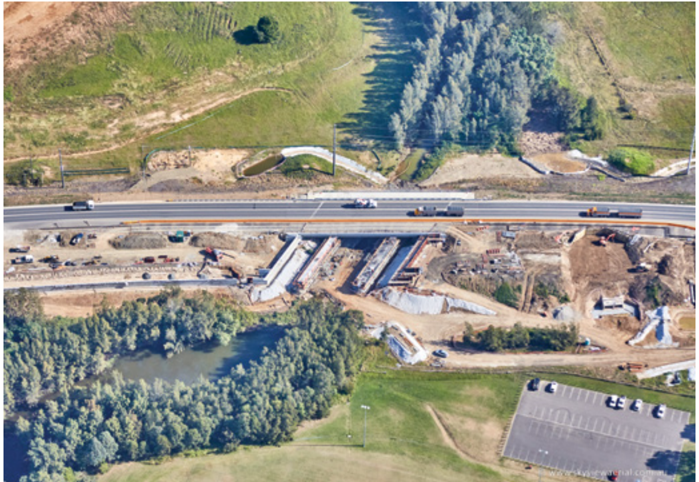
Work on the new northbound bridge over Narellan Creek, Harrington Park, May 2017
