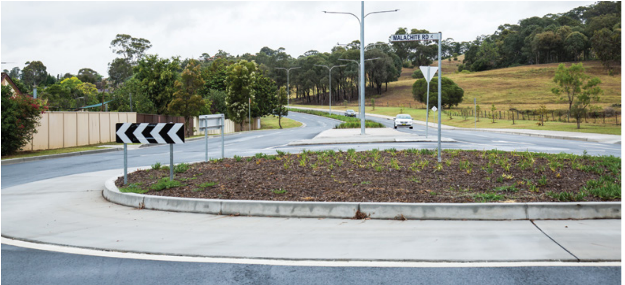
New roundabout on Eagle Vale Drive at Malachite Road, Eagle Vale looking south, December 2016
