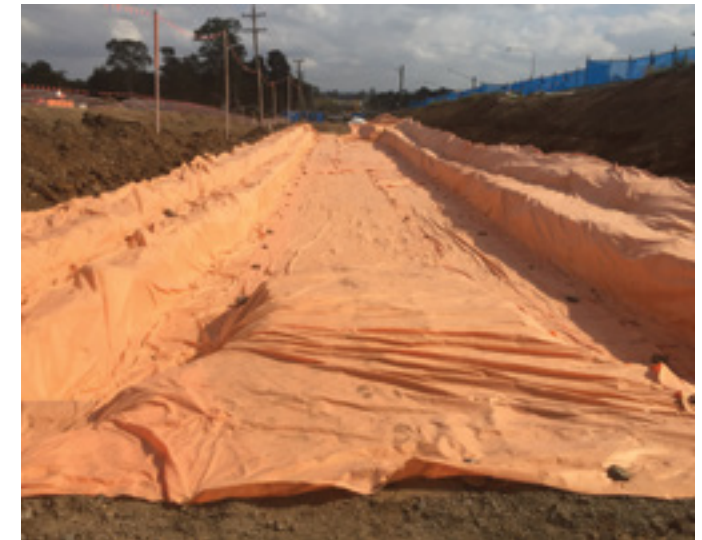
Bonded ACM encapsulation on the first stage of the Bringelly Road upgrade
