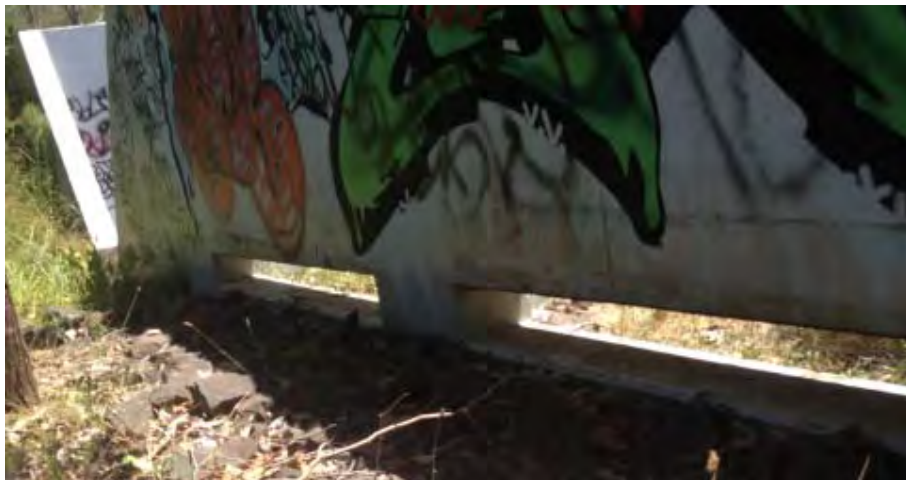
Figure 2-1 The horizontal slots in the v-notch weir structure
