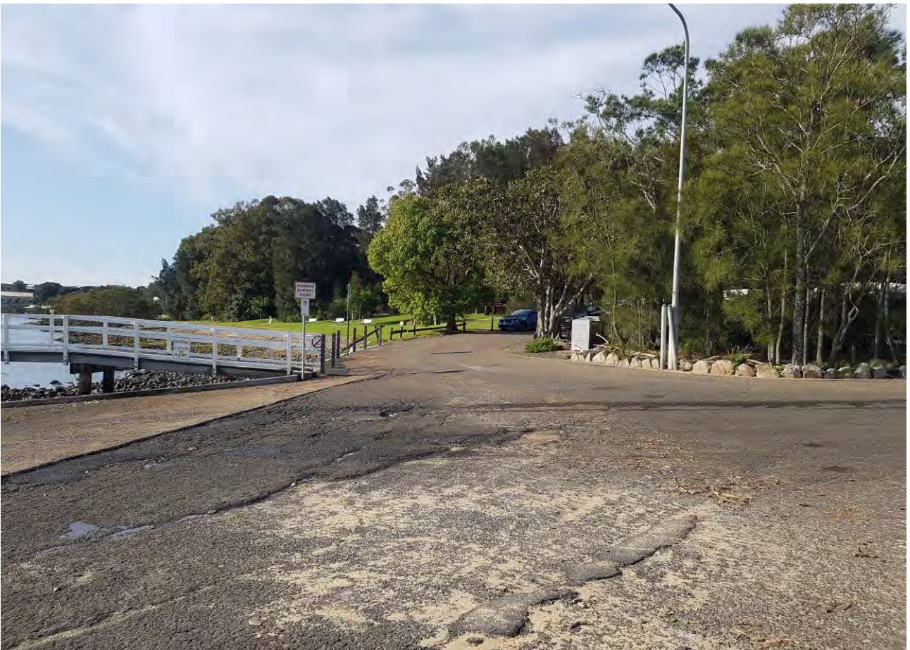
Figure 15: The commuter carpark terminates in a turning circle at the southernmost point of the headland
