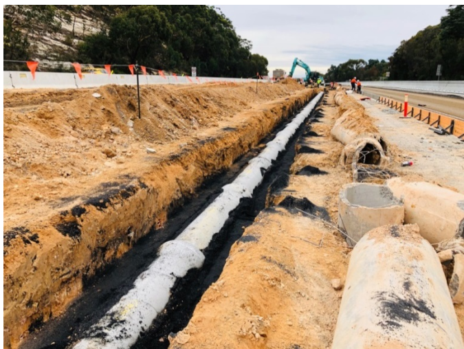
A total of 1.4 kilometres of stormwater drainage has been upgraded along the entire length of the project
