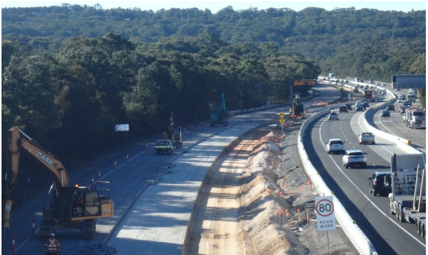
View north from Reeves Street overpass of the two northbound M1 lanes shifted across onto temporary asphalt in the median - July 2019
