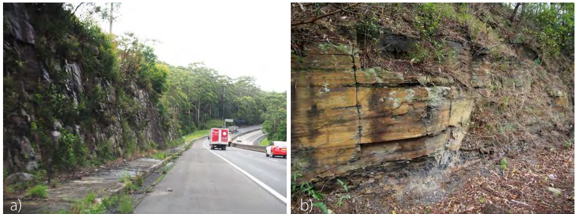
Figure 8 – a) Sandstone cutting with vegetation growing in weaker seams b) weaker stone and soil incursions
