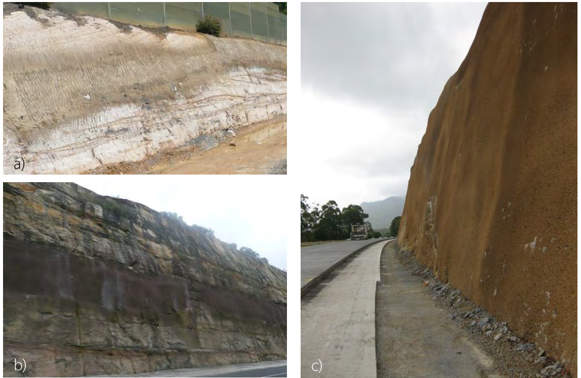
Figure 43 – Shotcrete treatments a) and b) depict seam treatments to sandstone cut face on M2 and the M1 Princes Motorway respectively. c) Depicts the treatment of an entire rock face and the issues associated with such a strategy with a relatively even and consistent finish to the face. This is an unacceptable outcome.
