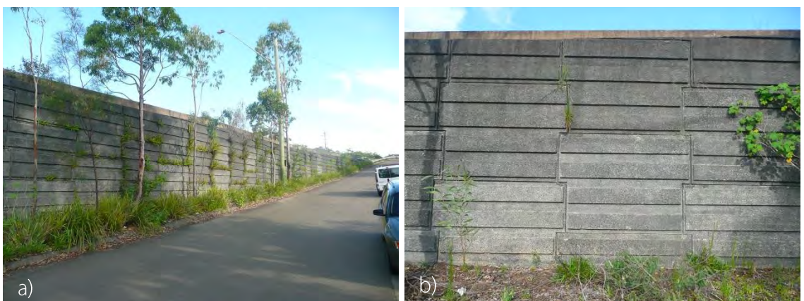
Figure 48 – a) and b) Exposed aggregate finish to Reinforced Earth wall below the Great Western Highway
