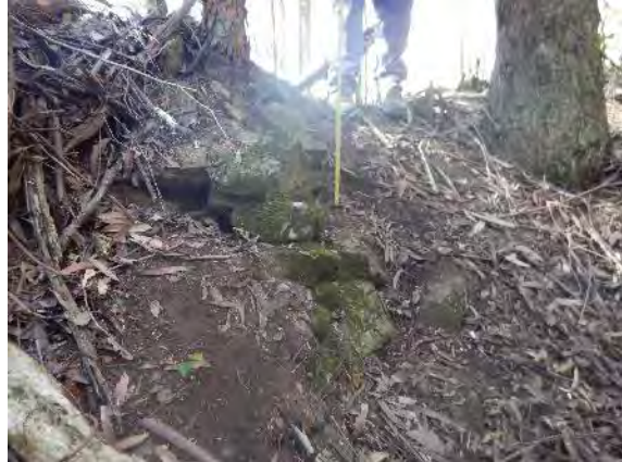
Figure 43: Sandstone retaining wall showing damage from vegetation, northwest aspect
