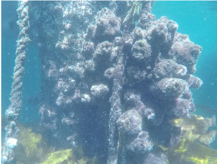
Figure 3-3: Typical communities and condition of vertical wharf piles in the study area
