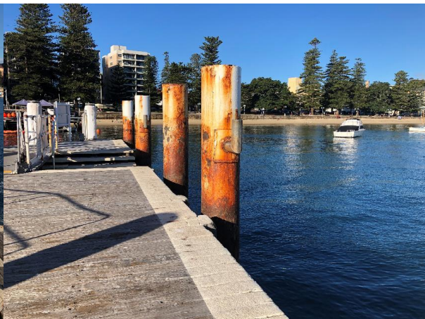
Figure 42 Corroded metal piles at the end of Wharf 3 (Artefact, 2021)
