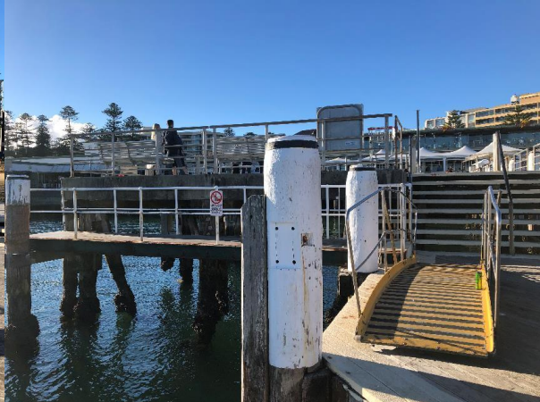
Figure 38 View towards steps leading down to Wharf 3 passenger area. Photo looking northwest (Artefact, 2021)
