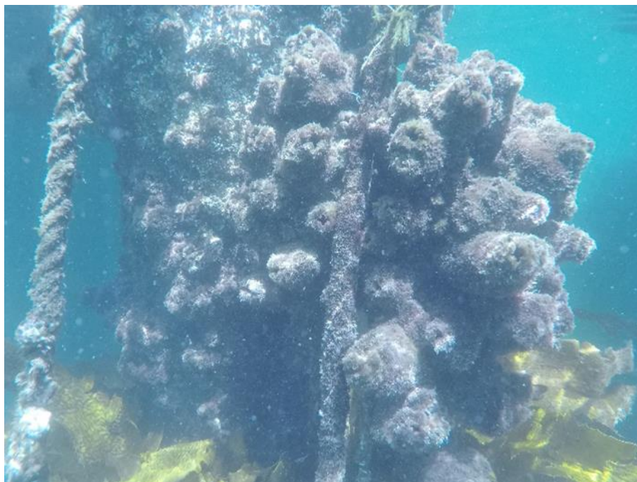
Figure 2-1 Typical communities and condition of vertical wharf piles in the study area
