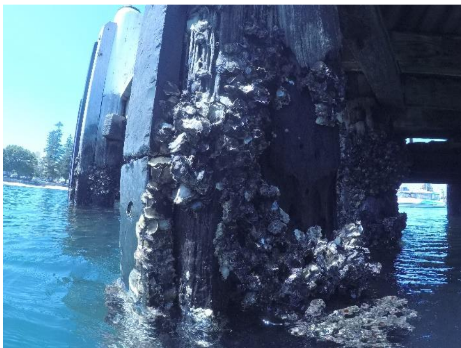
Figure 3-7: Typical communities and condition of intertidal timber wharf piles in the study area
