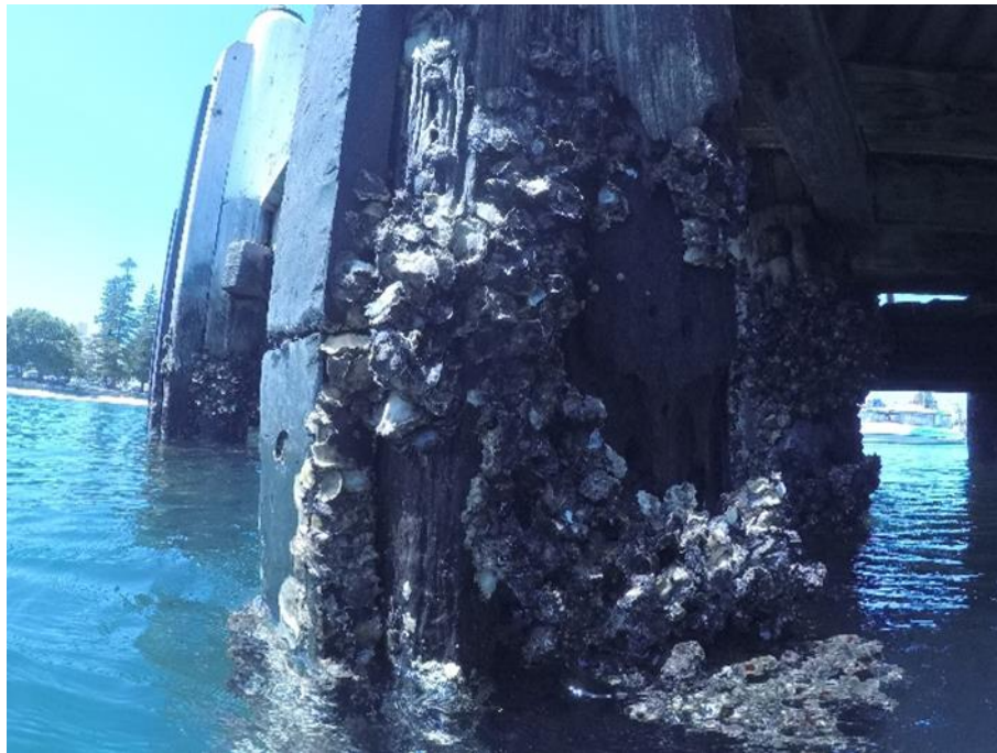
Figure 2-5 Typical communities and condition of intertidal timber wharf piles in the study area
