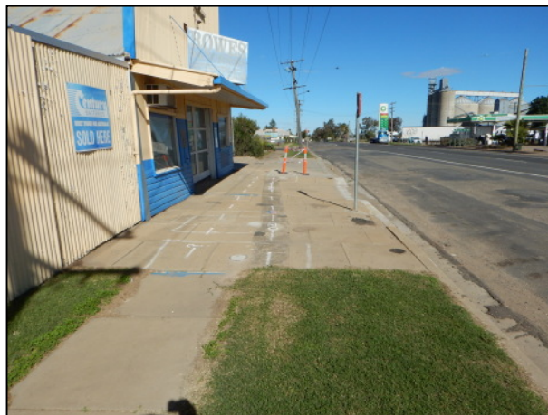
3. Overview of the LS Rowe Stock and Station Agents building and pavement, facing south.
