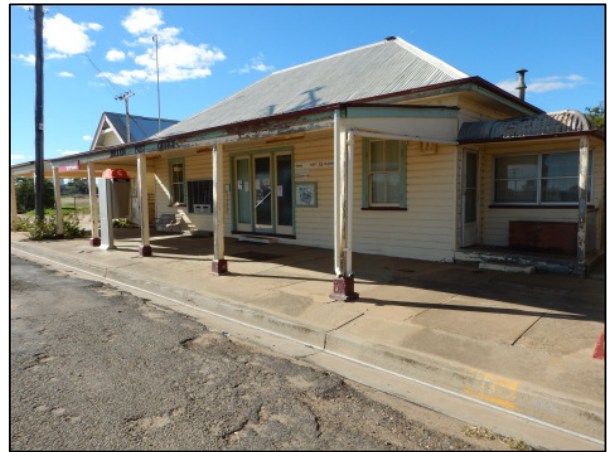
2. Overview of the Bellata Post Office building showing the building frontage and veranda over the pavement, facing northeast.
