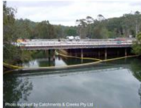
Photo 2 – Sheet piling used to form a dry work area with a floating silt curtain used as a sediment containment system
