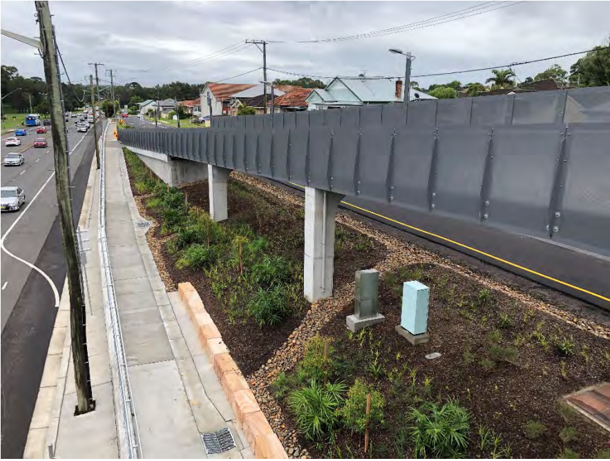
Photograph D.5 Drainage works and foot path under northern side of footbridge
