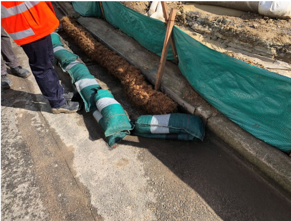
Photograph D.10 View of appropriate bunding and sedimentation controls implemented along Newcastle Road
