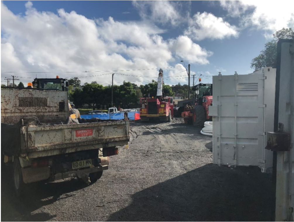
Photograph D.1 View of construction equipment, heavy vehicles and storage on site (Ancillary Facility)
