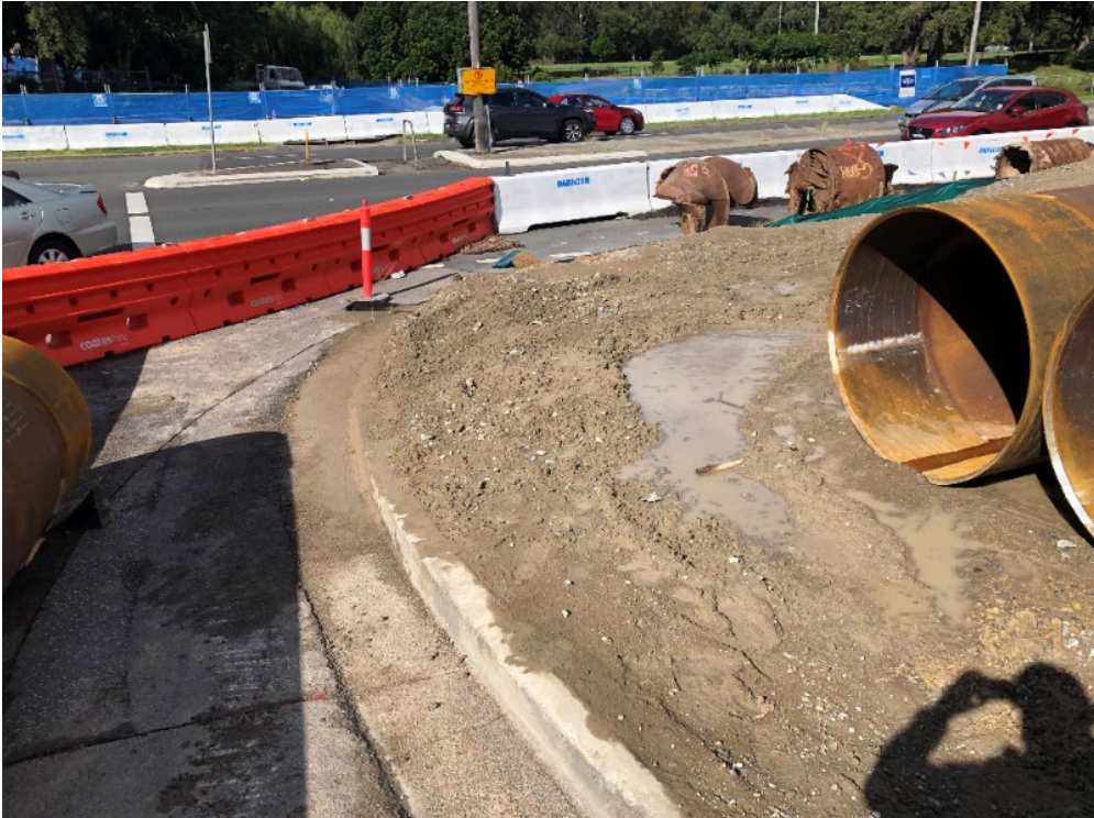
Photograph D.111 View of area where additional ESC required (Coles St / Newcastle Rd intersection)
