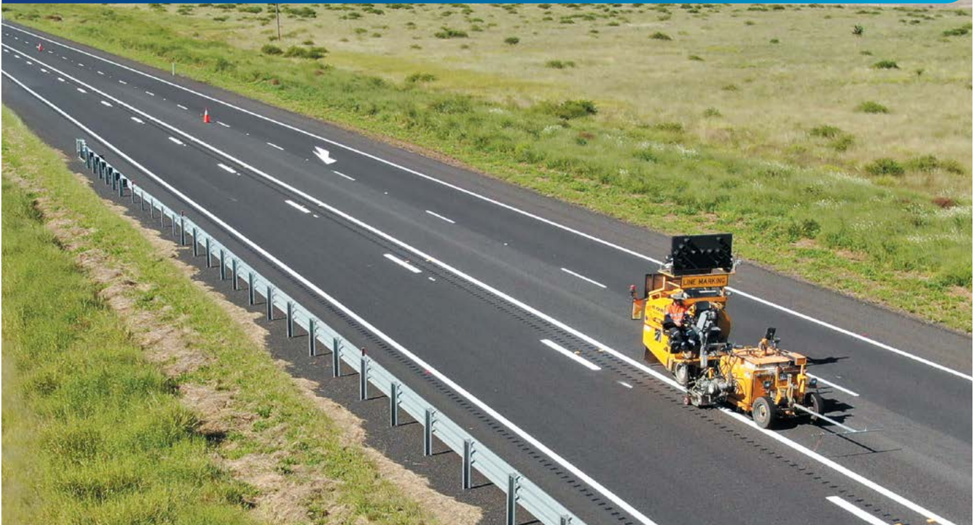
A section of the Newell Highway Mungle Back Creek to Boggabilla upgrade
