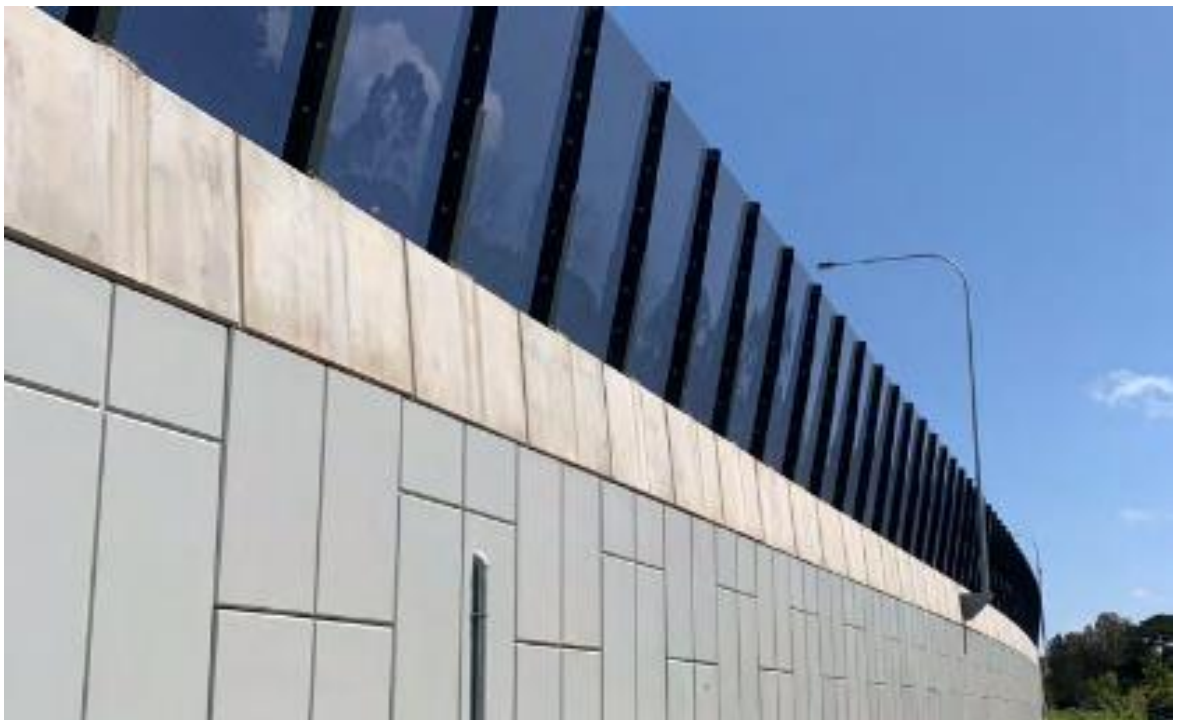
Figure 5.5 Image of acrylic safety screen with highly visual permeability (image also suitable for noise wall on the soil-wall section of bridge)
