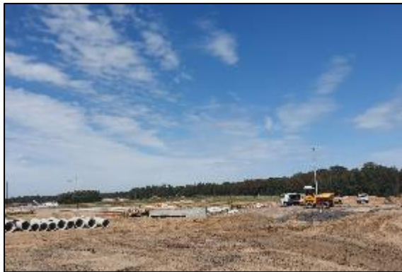
Plate 17. Construction activities within former Schofields Aerodrome, Eastern Creek in the background, facing south-west
