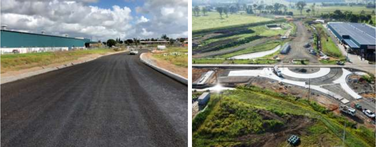
Figure 2 Seal and subsoils place on fill 2 (left) and construction of the new roundabout at Iolanthe and Through Street (right)
