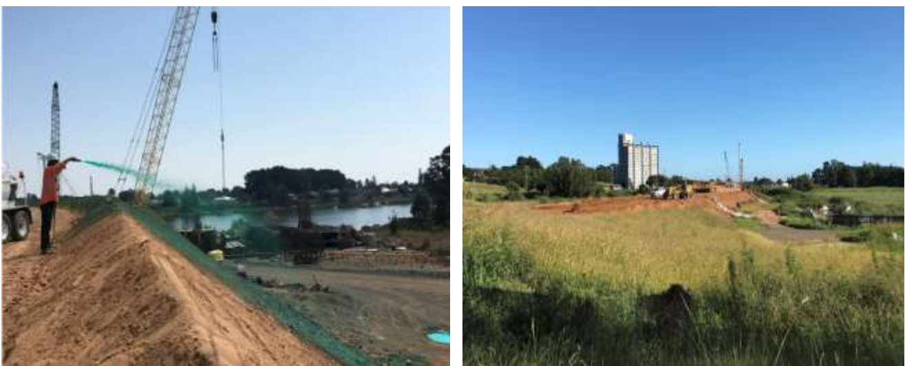
Figure 8 Polymer application to exposed dirt in South Grafton at Abutment A (left) and new grass growth at the Hydroseeded area in Fill 1 (right)
