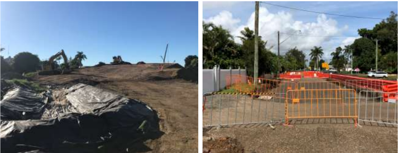
Figure 3 Fill placed at abutment B to pre-load level (left) and upgrades to local roads, Clarence Street, in Grafton being undertaken (right)
