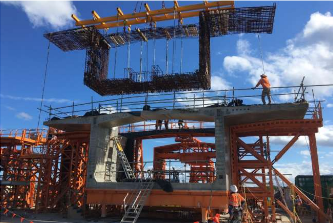
Figure 5 Pre-fabricated reo cage being placed into the mould with pre poured segment placed in front for match casting
