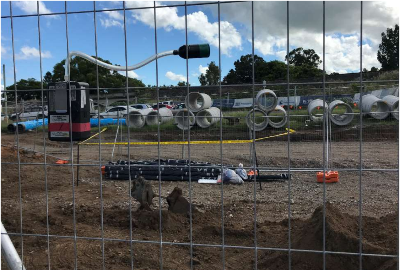
Figure 4 Removal of asbestos pipes from Pound Street, photo shows the pipes wrapped, exclusion zone around the area and air monitoring device on the fence
