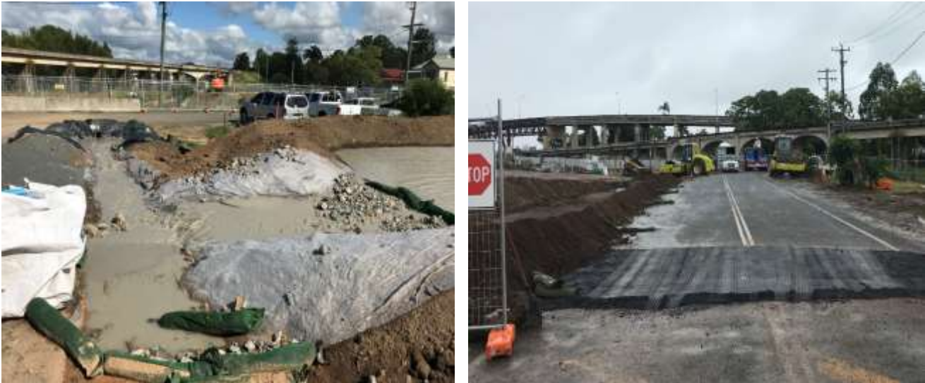
Figure 11 Controls installed to manage piling water during air lifts and pile pours in Grafton (left) and additional controls and drains installed along Kent Street, Grafton to manage potential dirty water run off (right)
