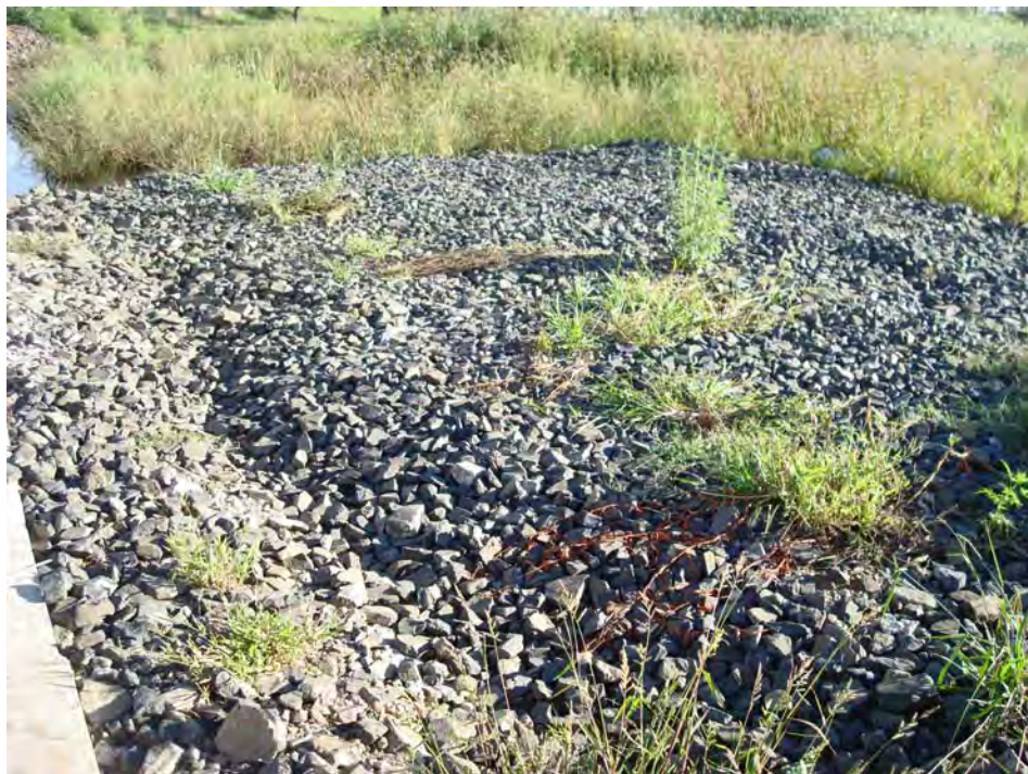
Photograph D- 8: Old working platform
