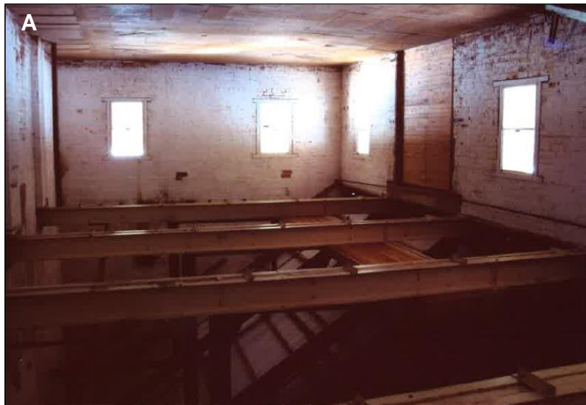
Plate 1: Interior of Gunnedah Maize Mill (Formerly Brunton's Flour Mill). Courtesy of Mr Stephen Dangerfield.
