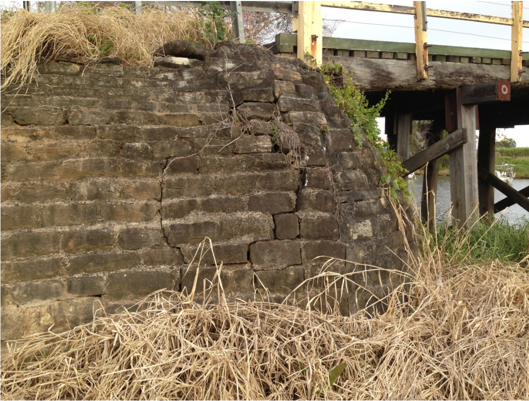
Photo 3: Dry-stone wall at northern abutment showing inferred settlement induced cracking.
