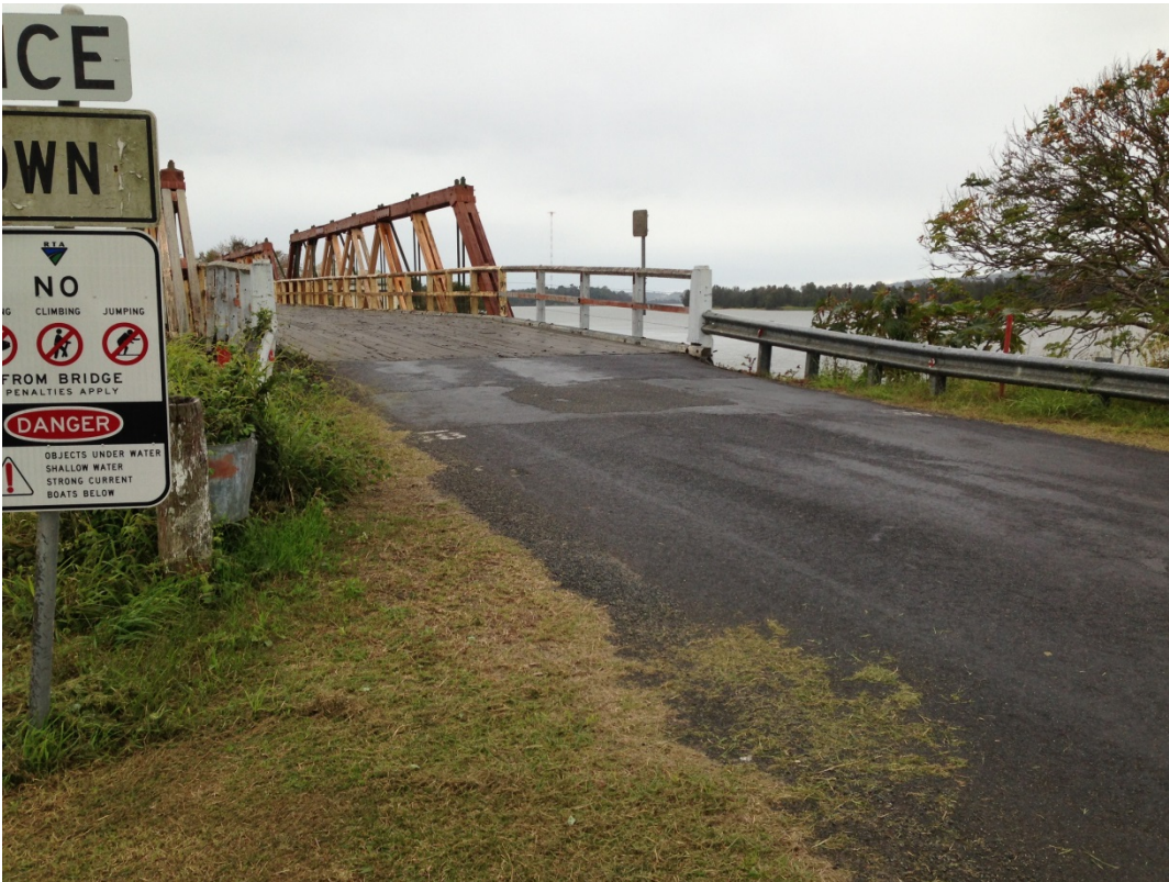
Photo 2: View at southern approach pavement/embankment showing evidence of settlement of the approach embankment.
