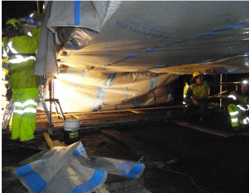
Plate 5.3 Effective plastic microbat exclusion installation at McFarlane Bridge, a similar structured timber bridge
