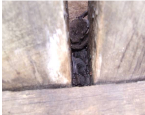
Plate 3.2 Large-footed Myotis roosting in bridge decking
