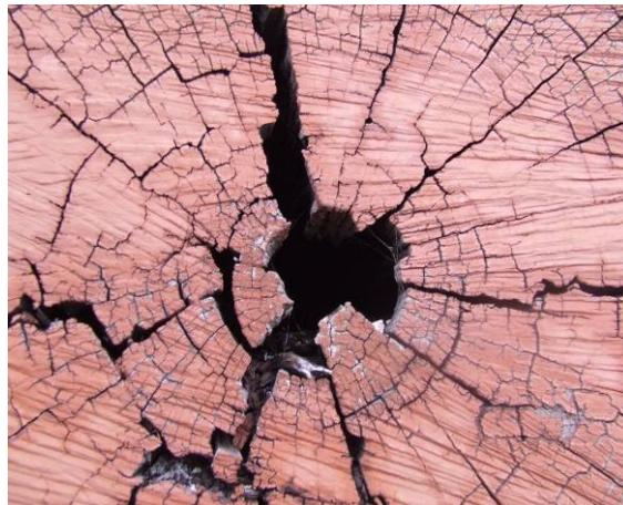
Plate 3.3 Cavity at the end of a rotted girder
