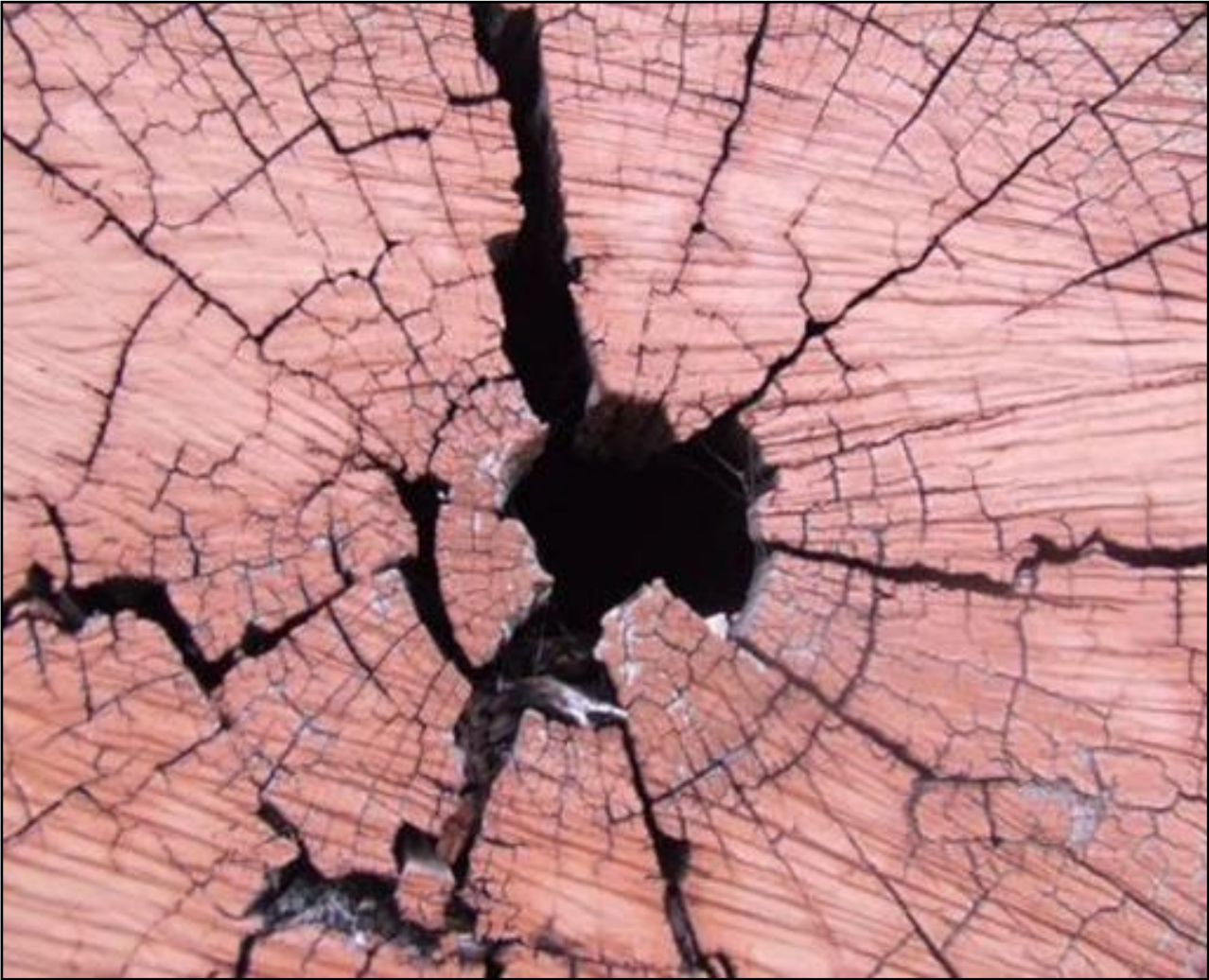
Plate 6.8: Cavity at the end of a rotted girder
