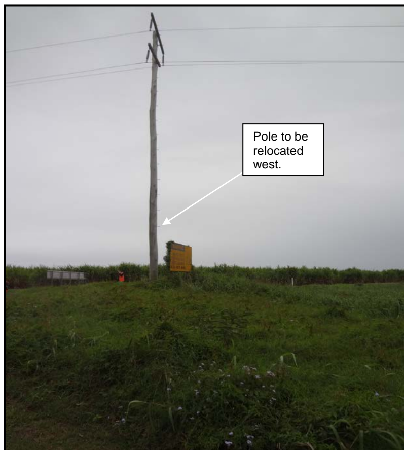
Plate 3.16 66kV pole to be relocated at the location of the southern approach
