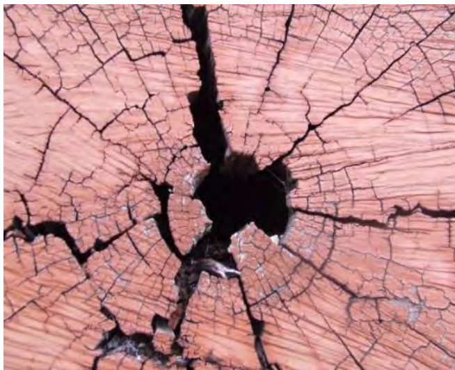
Plate 3.8 Cavity at the end of a rotted girder
