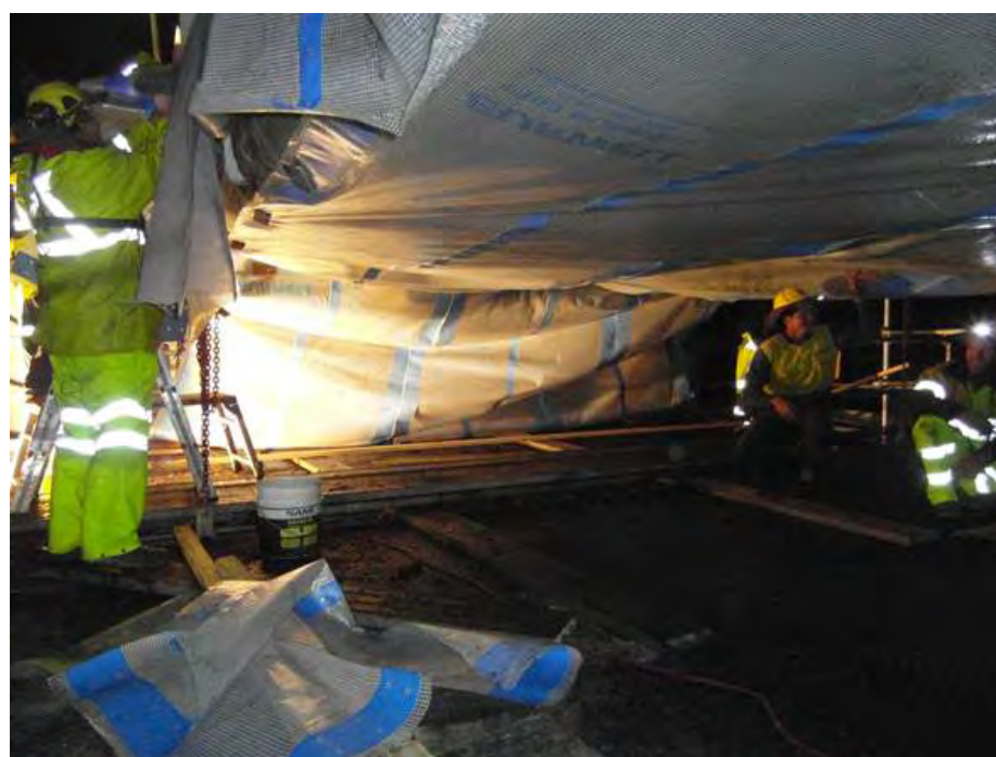
Plate 6.1 Effective plastic microbat exclusion installation at McFarlane Bridge, a similar structured timber bridge
