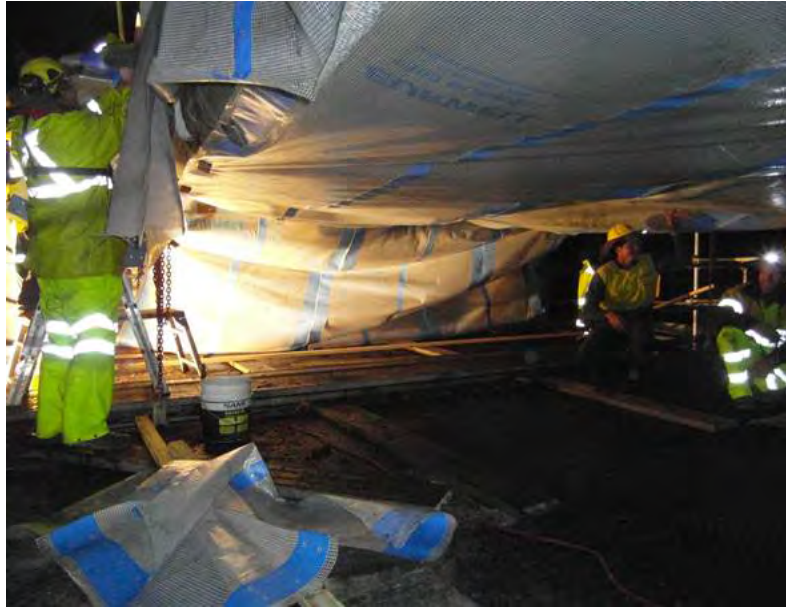
Plate 2.1 Effective plastic microbat exclusion installation at McFarlane Bridge, a similar structured timber bridge
