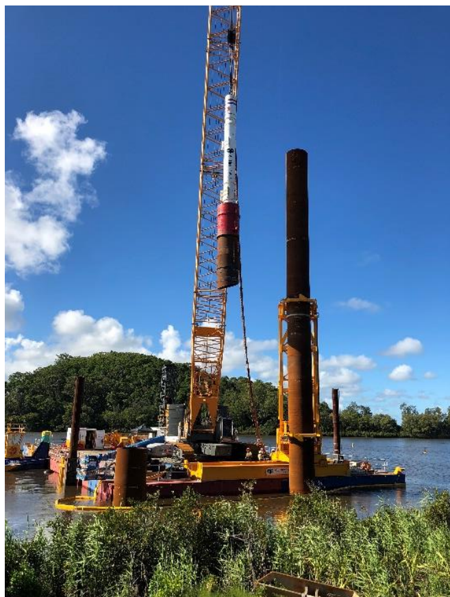
Photograph of crane, piling hammer, piling leader holding a pile in place
