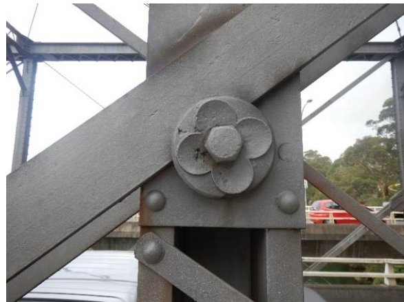
Figure 4.8: Detail view of cast iron rosette on the structure of the Nowra truss bridge
