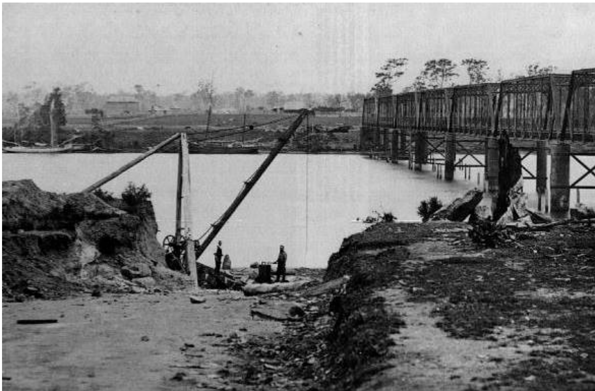
Figure 3.7: Workers near the Shoalhaven River and bridge, 1881. Photograph taken from north-eastern side of the river by Auguste Tronier, where the fisherman co-op is today. Note bridge approaches are incomplete. Source: Wollongong City Library
