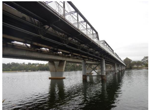
Figure 4.4: View from underside of Nowra Bridge, pedestrian walkway seen attached to the truss bridge
