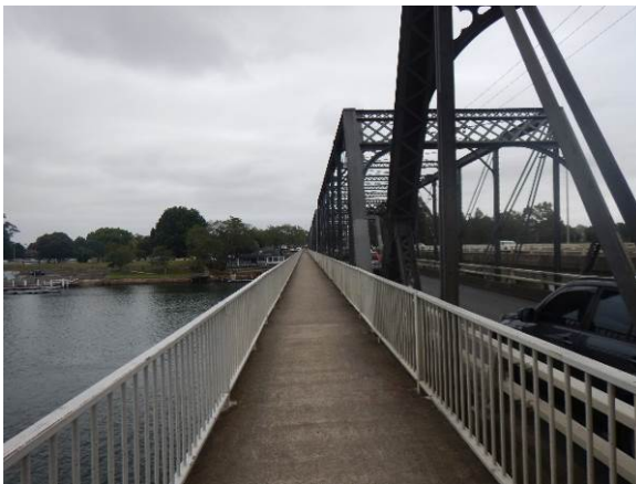
Figure 4.7: View south along the pedestrian walkway off the Nowra truss bridge (seen right)
