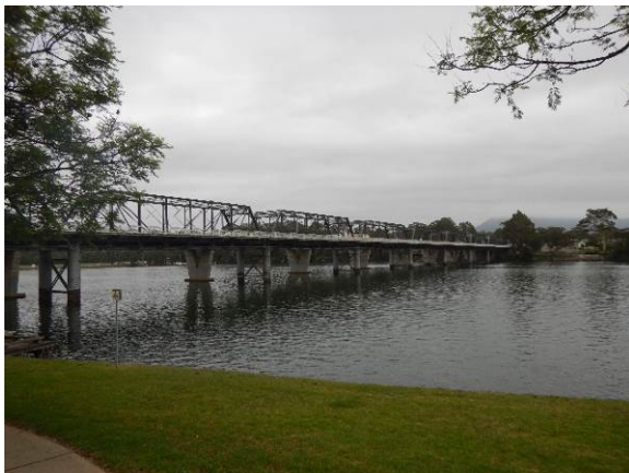
Figure 4.3: View north west across the Shoalhaven River to Nowra Bridge, pedestrian walkway seen attached to the truss bridge
