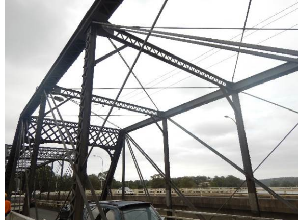
Figure 4.6: View of the Nowra truss bridge with northbound concrete bridge seen in distance
