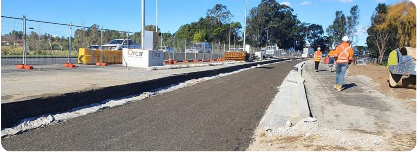
Pavement work on the Princes Highway between Bridge Road and Moss Street
