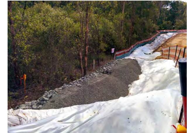
PHOTO 3 - EXAMPLE OF ROCK FILTER DAM AND SUMP
