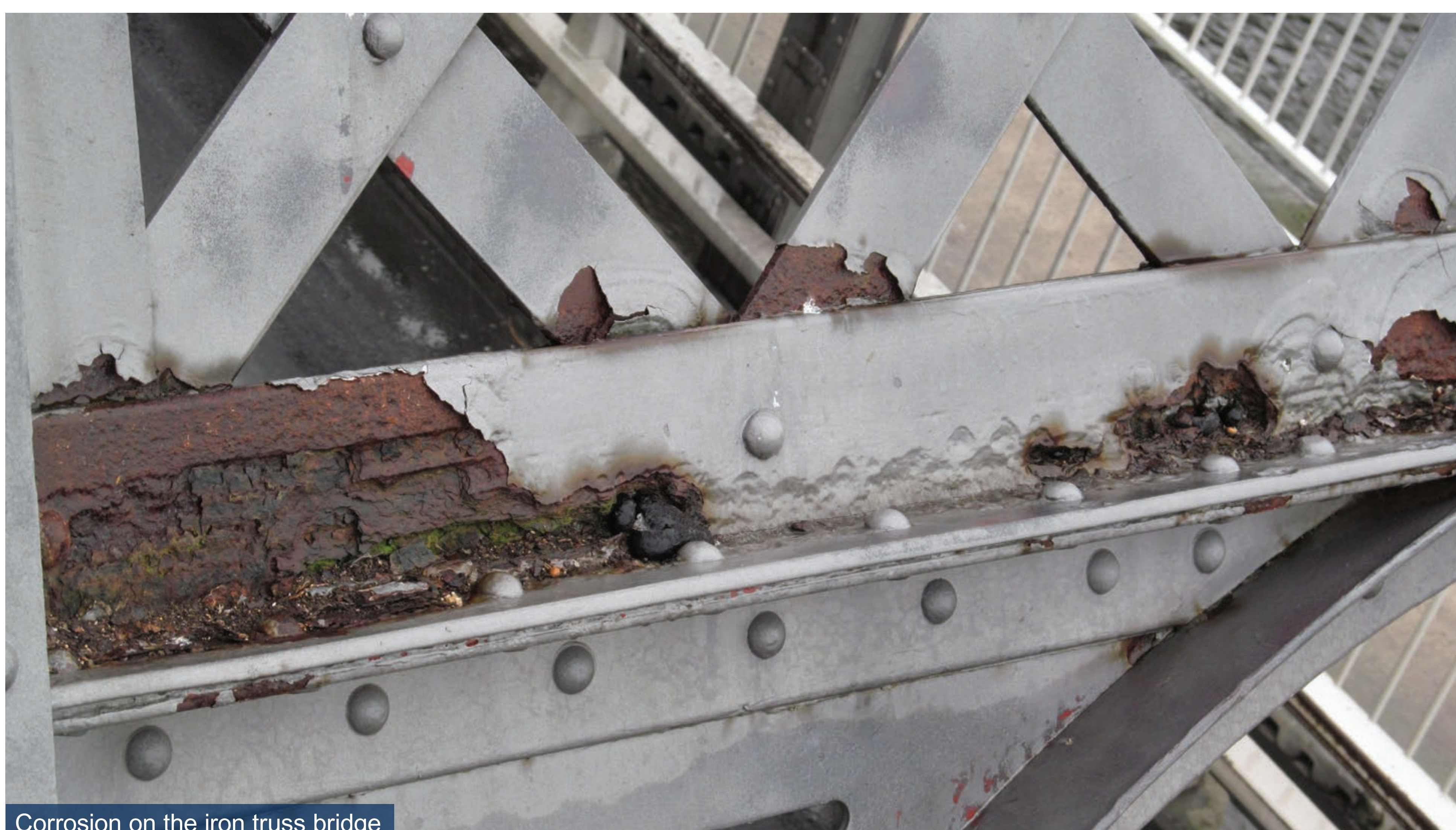
Corrosion on the iron truss bridge
