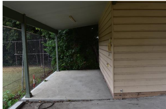
Figure 22. View south-east showing modern poured concrete slab and timber supports for c.1990s shed.
