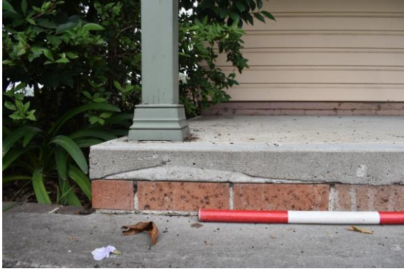
Figure 25. View of poured concrete slab, brick foundation and timber support associated with the c.1990s shed.
