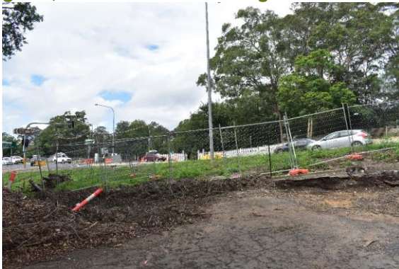
Figure 21. View south-west from c.1990s shed towards Princes Highway and Nowra Bridge Relocation works.
