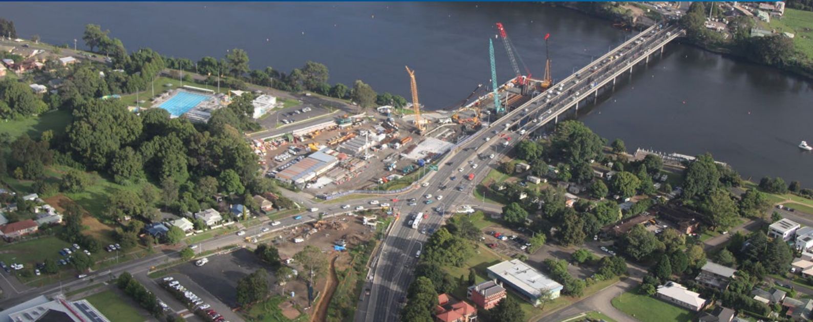
Casting yard and piling on the southern side of the Shoalhaven River
